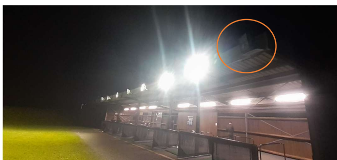
Figure 10 - Existing range lighting system failed light
