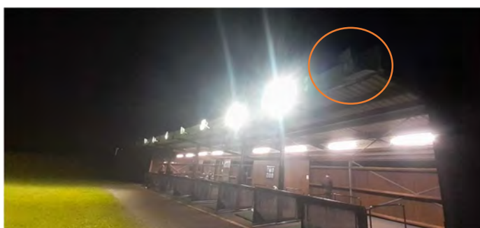
Figure 10 - Existing range lighting system failed light
