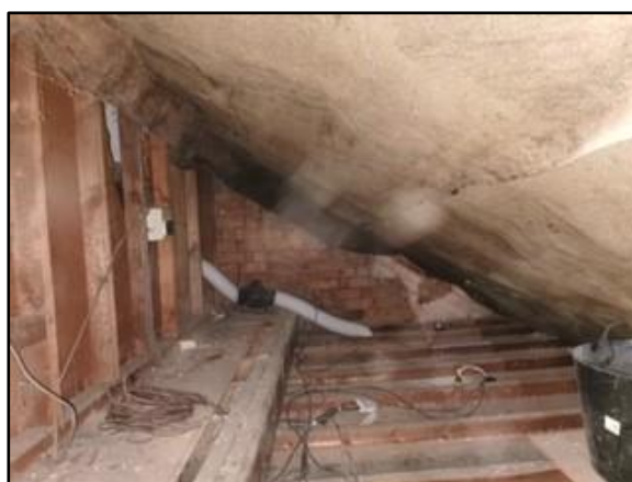
Plate 4: The void at the rear-facing (western) eave.
