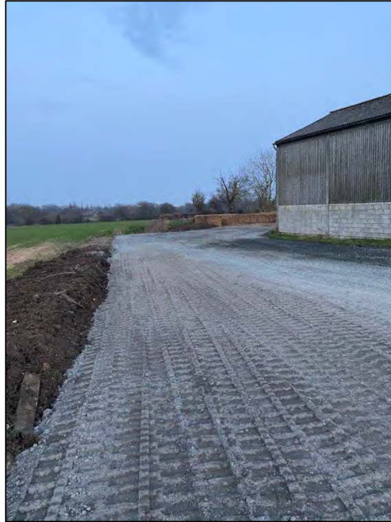
Photograph 9: The northern side of the barn, with Type 1 MOT hardcore track and countryside beyond.
