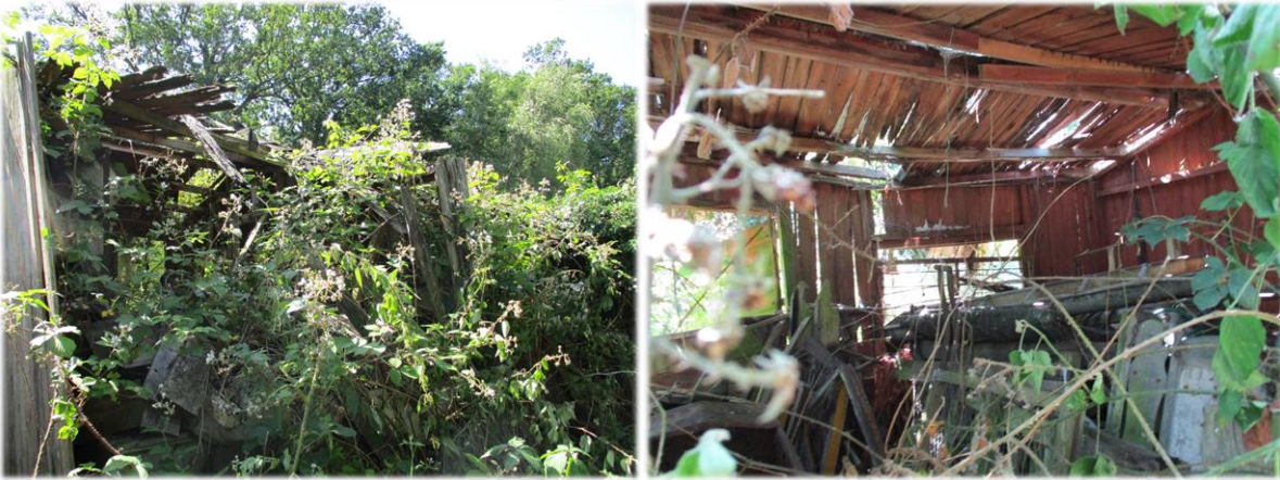
Dilapidated wooden shed covered in bramble
