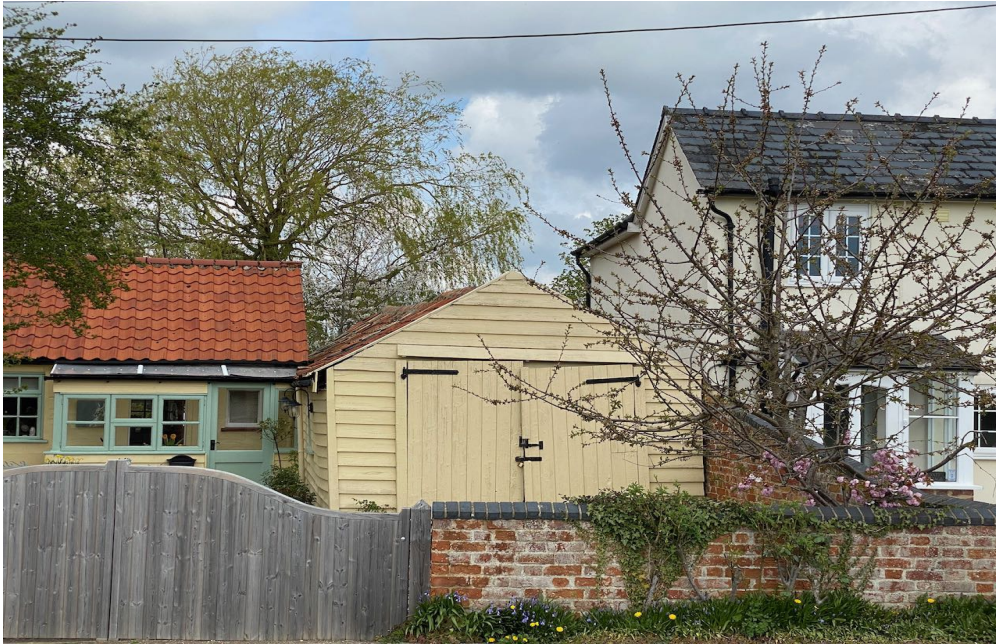
In the last 12 months alone, the timber outbuilding wall has collapsed a further 100mm
