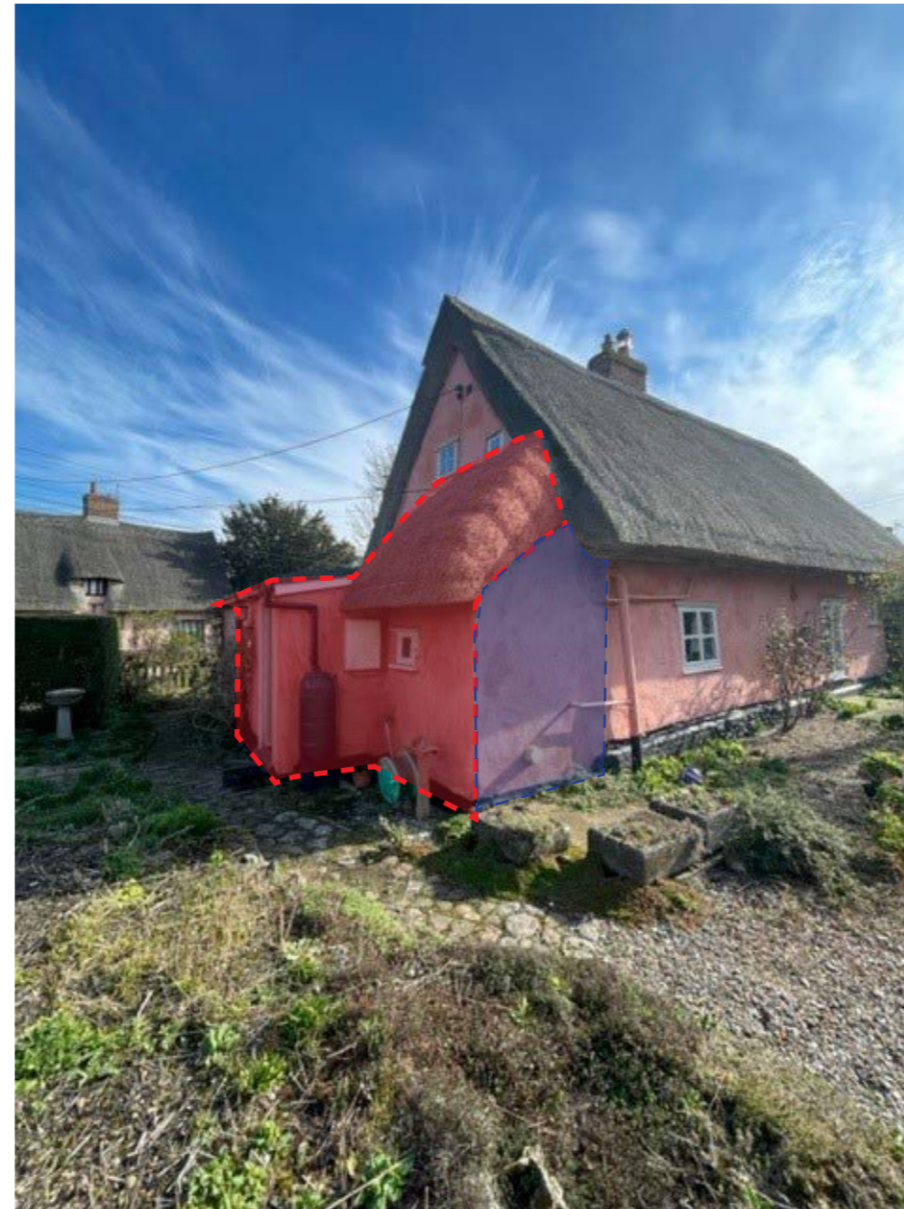
View 1- Kitchen Extension and Thatched roof to be replaced with reclaimed Terracotta Tiles. Structural beams untouched.
