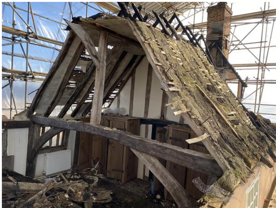
Figure 7: View looking south east showing open crown-post truss and timber mullion window in main chamber
