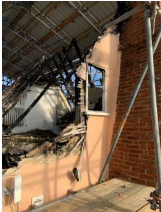
Plate 19. Damaged timber framed gable wall.
