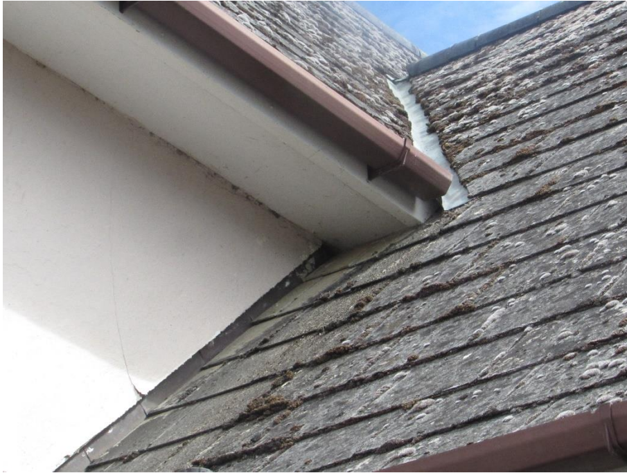
Plate 3 – Lead flashing on the valley of the south-western elevation of the house, small gap between lead flashing and soffit
