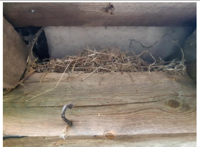
Photo 12 Northern room in garage Remains of passerine nest in wooden frame
