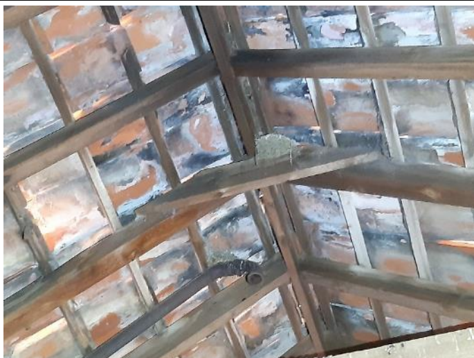
Photo 11 Interior of pantile roof, showing gaps, absence of roofing membrane and swallow nest adjacent to ridge
