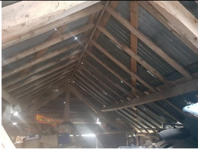
Upper floor of the barn. Tin sheets resting on a timber frame. Skylights along the length of the roof make the space light.
