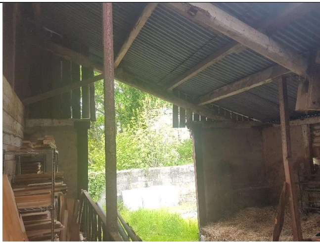
Lean-to extension at the north east facing elevation. Blockwork walls and tin roof.
