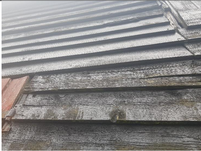
Board cladding detail. The boards do not provide suitable crevices for roosting bats and are not attached to anything behind.
