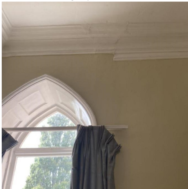
view of cornice return from corridor. Modern angled partition to the centre.
