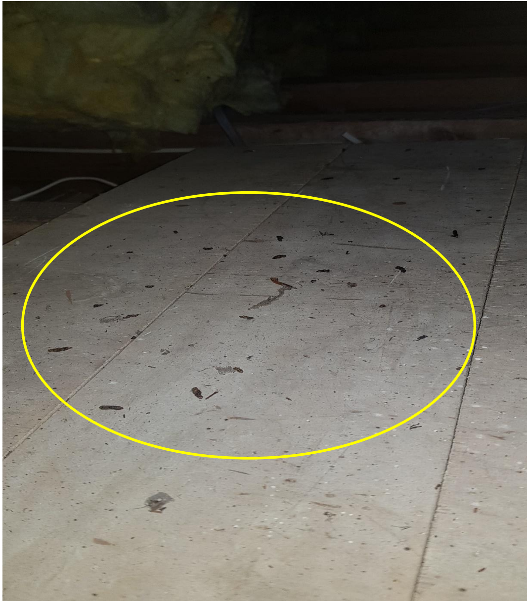
Picture 6: Showing the bat dropping on top of the floor boarding
