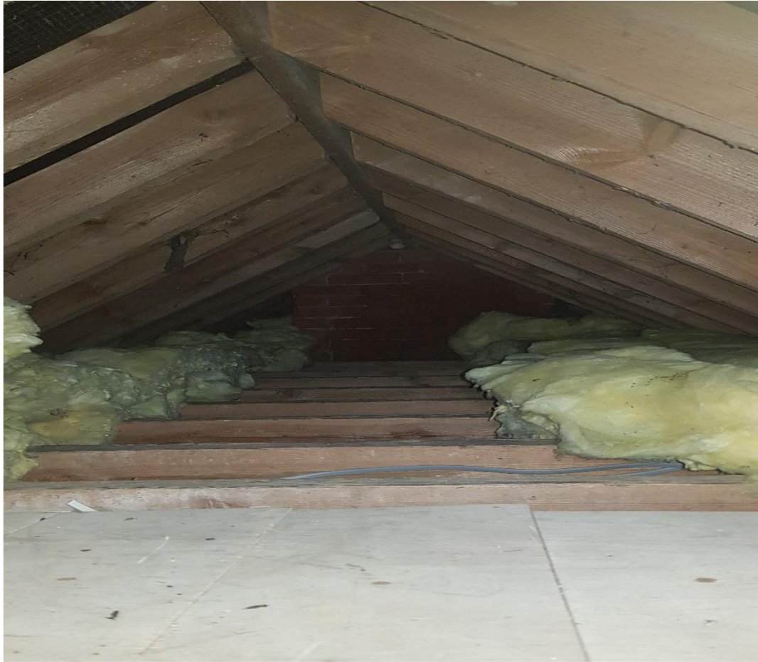
Picture 5: Showing the internal roof space of roof space 1 and 2 both very similar
