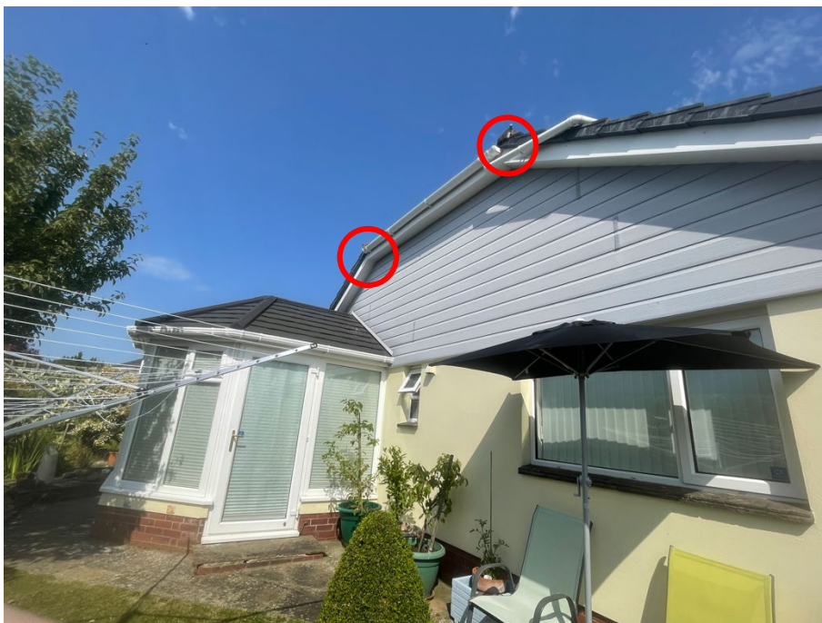
Photo 4: South elevation showing bird nesting locations.
