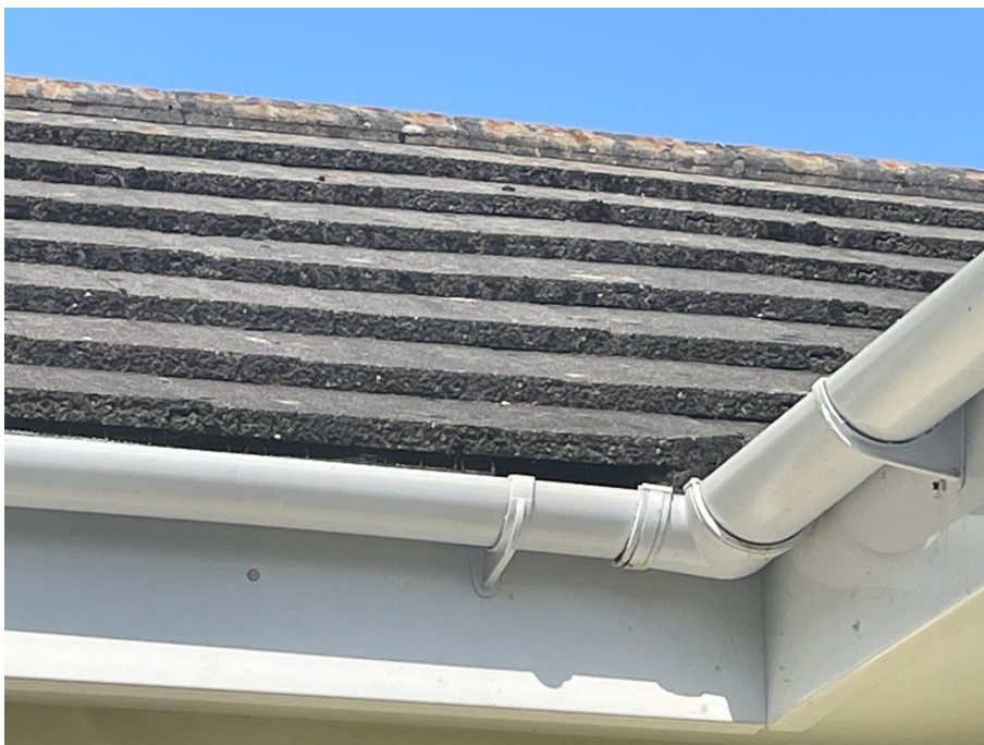
Photo 6: Lifted tile on east elevation of extension.
