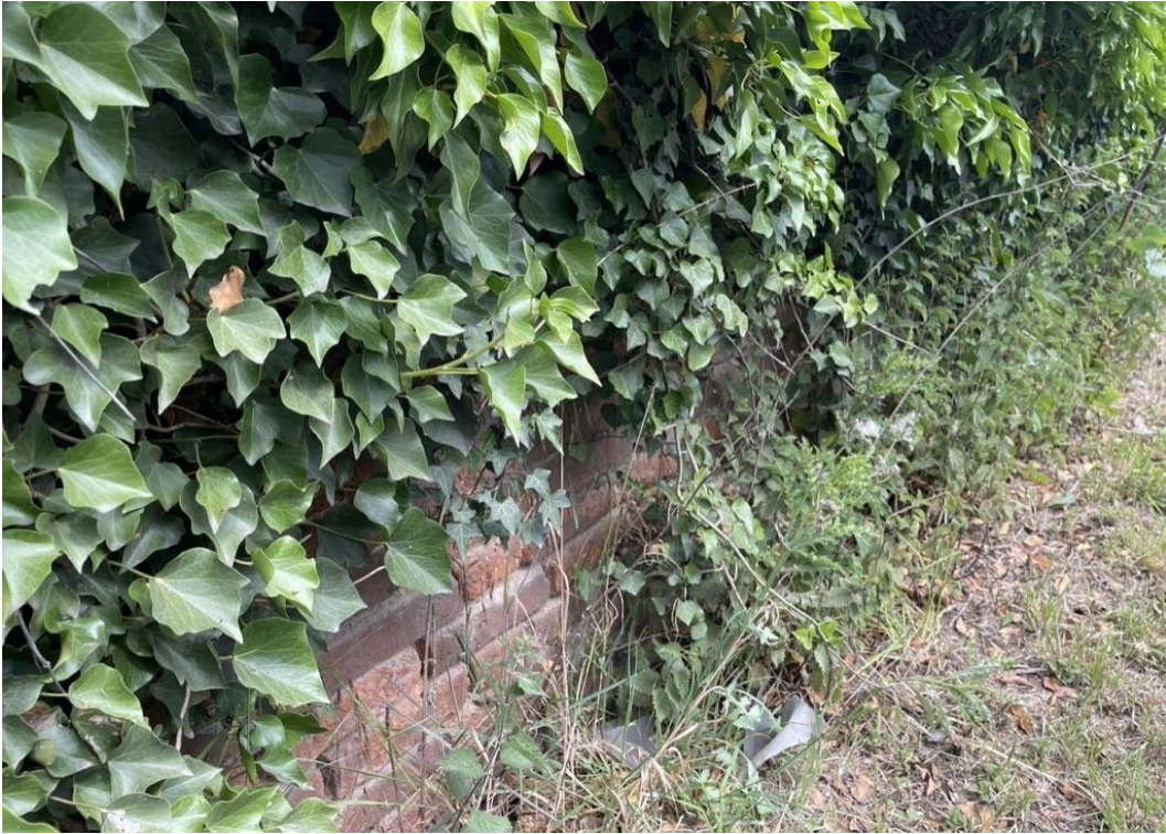
Photograph 13: Brick wall and ivy which forms the western end of the south boundary
