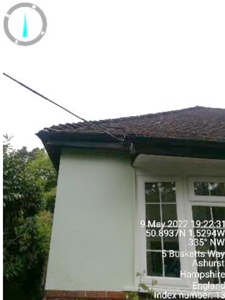
Photograph 11: View of the notable lifting of tiles on the south-west corner of the property.
