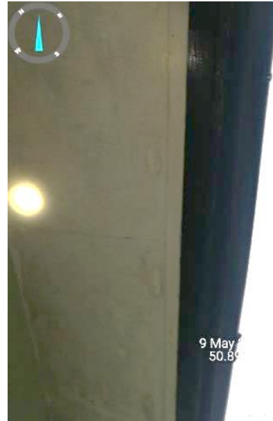
Photograph 8: View of soffit with gap between soffit board and fascia board.
