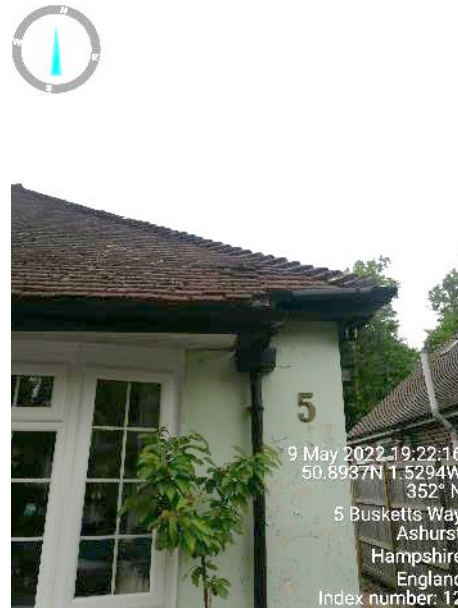
Photograph 10: View of the notable lifting of tiles on the south-east corner of the property.
