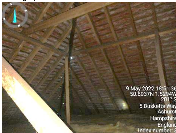
Photograph 3: View of loft with light emitting from ridge line evident.
