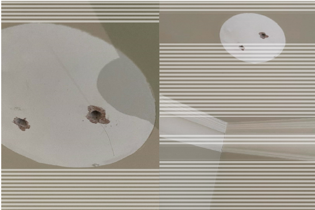
Appendix 2: Ceiling Plaster in Master Bedroom
