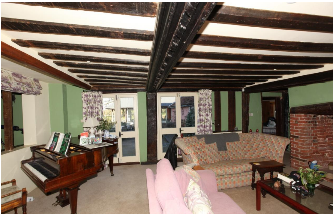
Illus. 10. The rear wall of the hall showing exceptionally large studs of some 9 inches in width to the right of the high-end window, which is now occupied by French doors. The common studs of the high-end bay to the right are neatly chamfered and stopped, but those of the low-end bay to the left are entirely plain.
