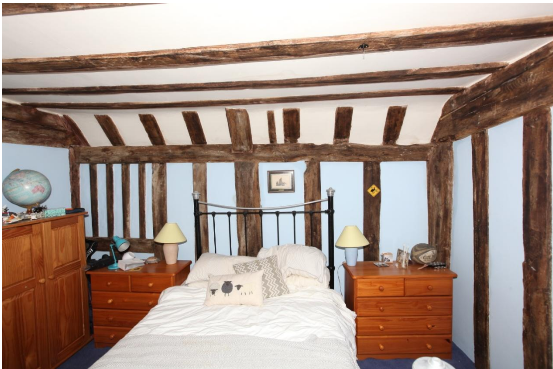
Illus. 20. The northern wall of the parlour chamber (bedroom 1) showing the principal rafter of the A-frame principal roof truss in the centre and an intact original window of chamfered mullions to the left. The truss is shown in illustration 24 and the window in illustration 21.
