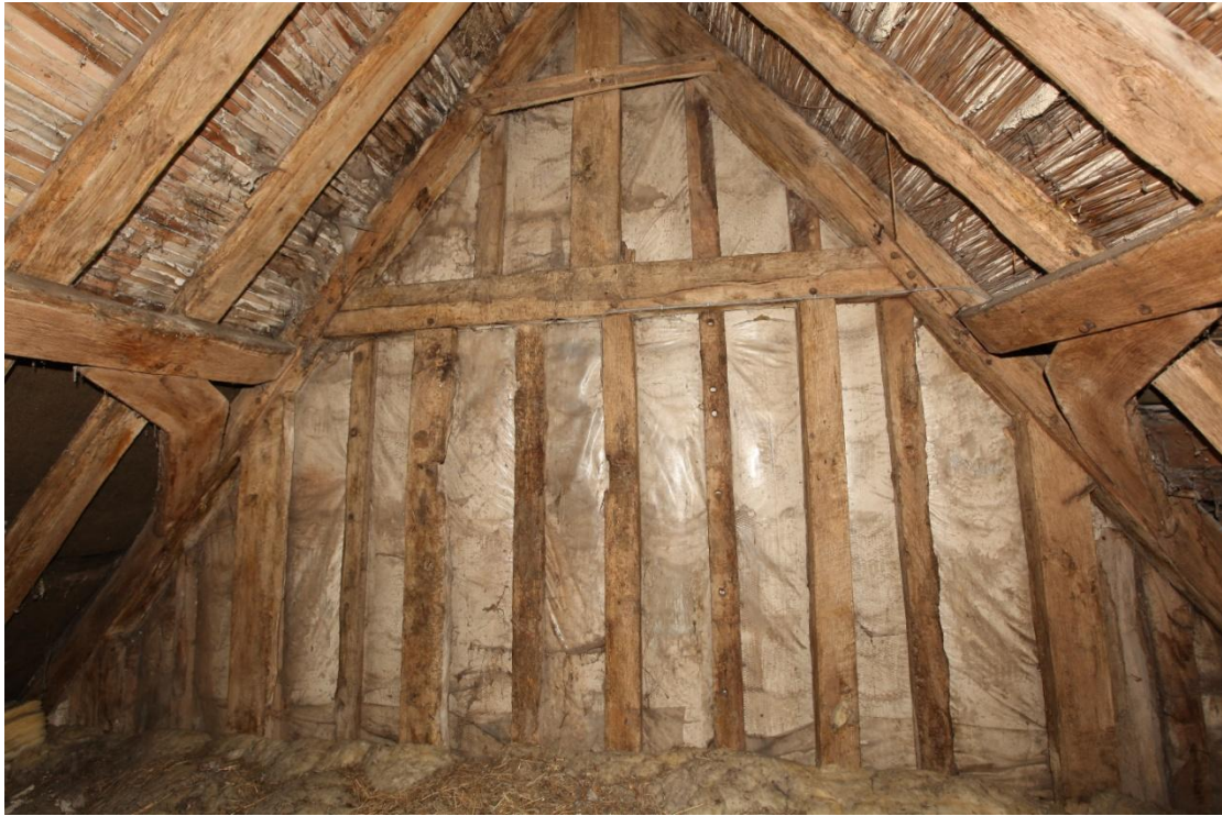
Illus. 25. The framing of the eastern roof gable in illustration 24, with narrow inserted studs between the wider originals which are pegged to the horizontal collar. The collar of the eastern gable is cambered and lacks stud mortices. Two mortices for diamond window mullions are visible to the left of centre, with corresponding pegged and housed sill mortices beneath. The window aperture respects the equal spacing of the studs and it was probably inserted along with the attic floor later in the 16 th century.
