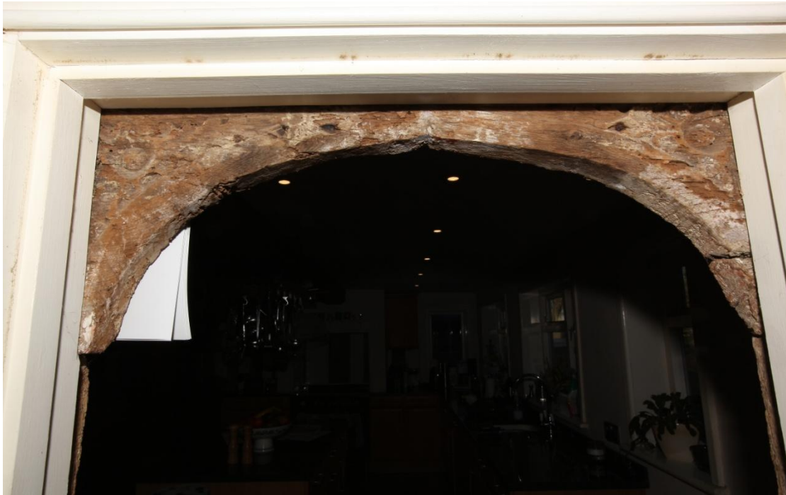
Illus. 13. The foliate-carved spandrels of the parlour door, seen from the Georgian dining room to the south (i.e. to the left in illustration 31). Traces of old red ochre pigment are visible beneath the later whitewash, giving another possible explanation of the property's name.
