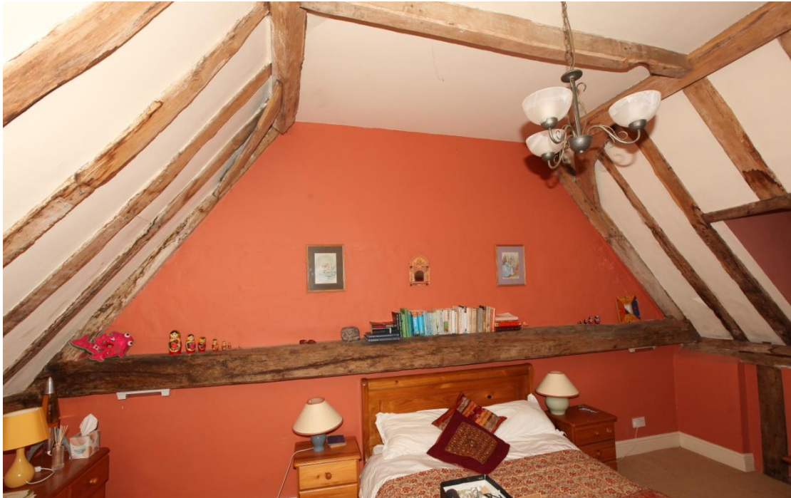
Illus. 23. The western gable of the 16 th century building (bedroom 3). The floor level is higher here than at the eastern gable (illus. 19) as the ground-floor ceiling joists have been raised, apparently to match the Georgian ceilings and accommodate the sash window in illus. 2. The tie-beam contains mortices in its lower surface but not its upper, suggesting the roof gable may have projected slightly in the manner of a jetty.
