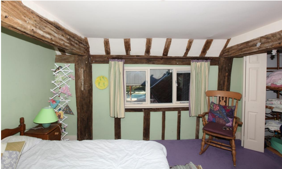
Illus. 17. The northern wall of the hall chamber in bedroom 2 showing the central open truss on the left and that adjoining the chimney bay on the right. Both preserve pegged mortices for missing arch-braces with a distinctly Tudor profile. The sloping flue of the original chimney would have been visible from this space initially. The roof-plate above the modern window contains mortices for diamond mullions as shown in illus. 18.
