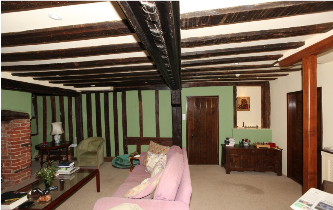
Illus. 9. The front wall of the Tudor hall, which now adjoins the Georgian range. The expensive, closely-spaced studs indicate the building's high status, but those of the upper storey, unseen by visitors, were far less close. This anomaly was originally disguised externally by render. The horizontal timber to the left of the door is the thick sill of a projecting, oriel window. Part of the original arch to the cross-passage entrance survives in the narrow door jamb to the right of the present door, but the hall's corner post has been moved 18 inches to the left of its original position to enlarge the service bay.
