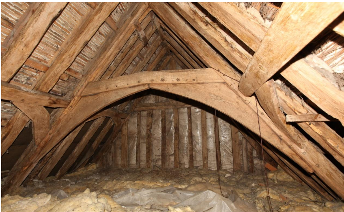
Illus. 24. The open truss of the fully wind-braced butt-purlin roof above the parlour chamber, with the eastern gable in the rear. An identical truss with an arch-braced, cambered collar survives in the centre of the hall chamber, with a flat, unbraced collar to the west of the chimney bay and another in the closed truss against the service bay. There is no principal truss to the east of the chimney bay. The first-floor ceilings are insertions, and this roof was exposed to the upper storey initially. Impressive as it seems, it may have been regarded as utilitarian given the plain mullions in the hall chamber.
