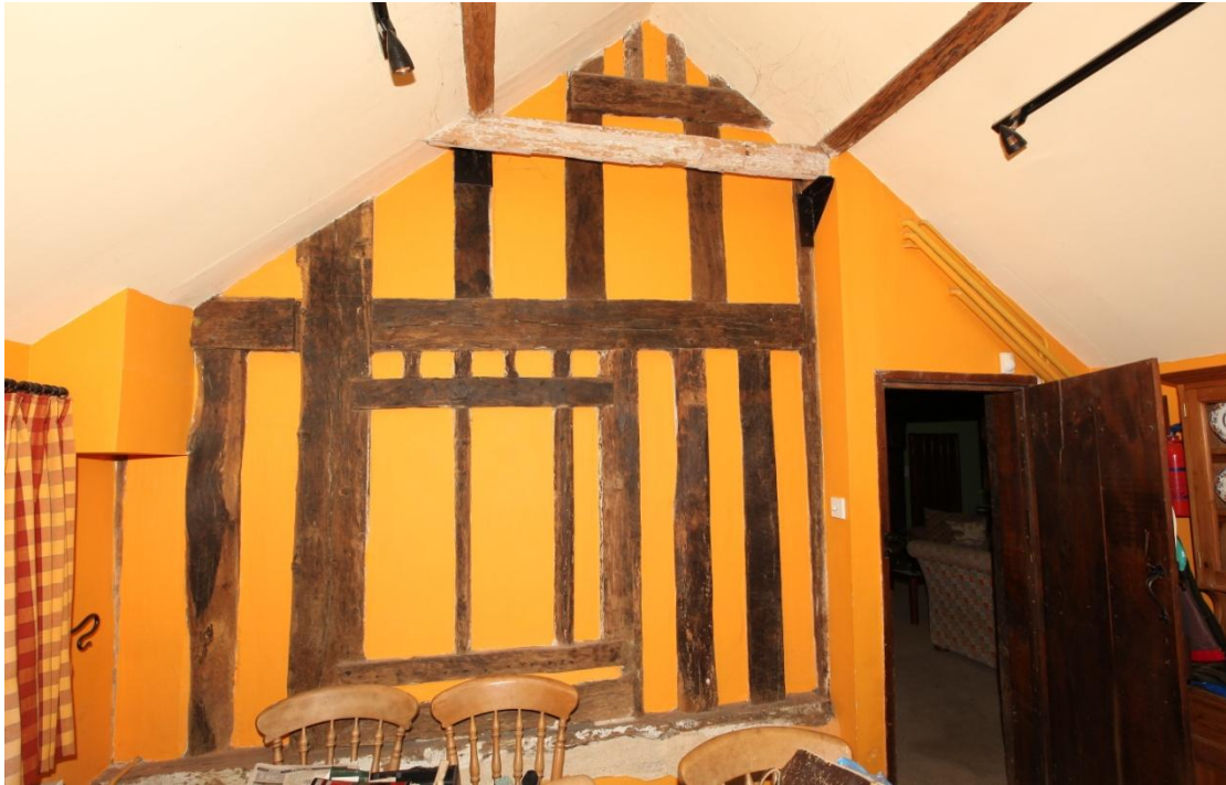
Illus. 15. The rear wall of the parlour, seen from the ostensibly early-19 th century brick service range to the north. The central post lies to the left with a ground-floor window to the right. Four original chamfered and pegged window mullions survive above the nailed lintel of a smaller, later window, and the original weathered sill overlaps the post and jamb beneath the later sill. A similar weathered lintel of the first-floor window in illus. 20-21 is visible at the roof apex. Two original mullions have somehow survived within the smaller window. The walls studs are not weathered, with their saw marks still well preserved, and the disparity between the closely-spaced ground-floor timbers and their widely spaced counterparts above would not have been visible.
