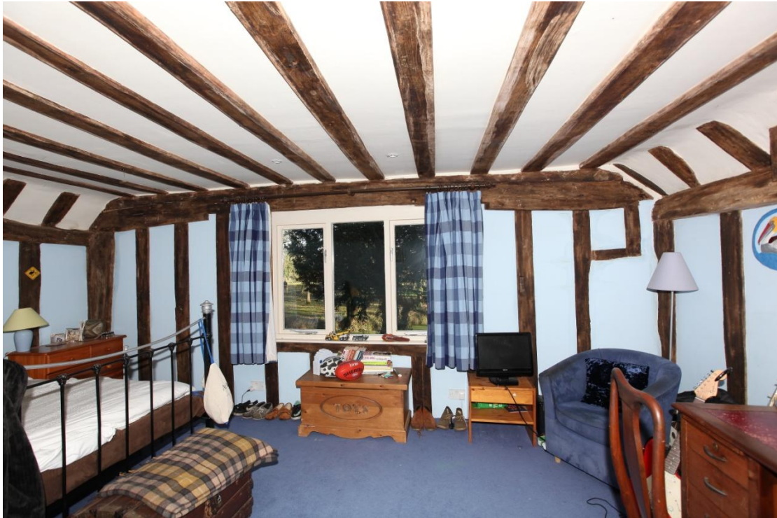
Illus. 19. The eastern gable of the parlour chamber with late-20 th century casements in the position of the central window and the intact lintel of an original garderobe (privy) adjoining the corner post on the right. The back of a mortice for the external cupboard-like projection is visible in the adjacent stud to the left. The lintel is pegged at both ends and is just 12 inches long, but the jambs were probably curved to widen the aperture.
