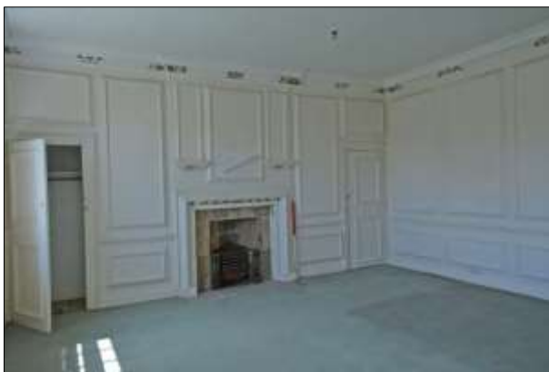
Plate 38: F3: west wall
