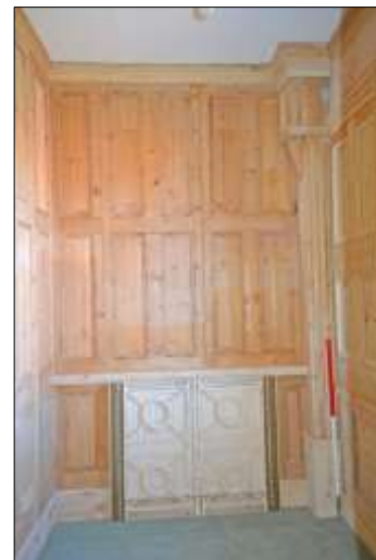
Plate 47: F6: west wall
