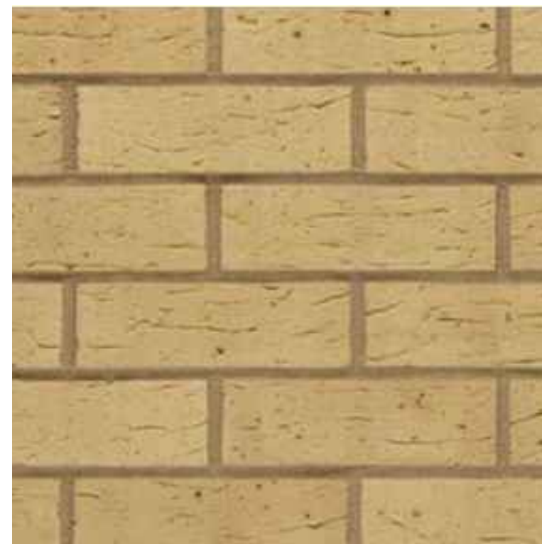
01. Ibstock Brick Nostell Royston Golden Buff (Brick arches to new window openings)
