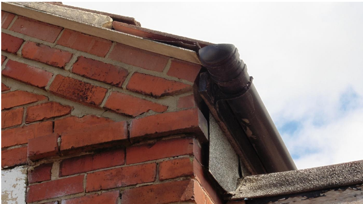
Photograph 8: Evidence of features such as the missing bedding mortar of some end tiles, leading to the exposed timber of the roofing frame, as well as gaps behind the bargeboard and behind a section of felt, all located on the south-western corner of the village hall.
