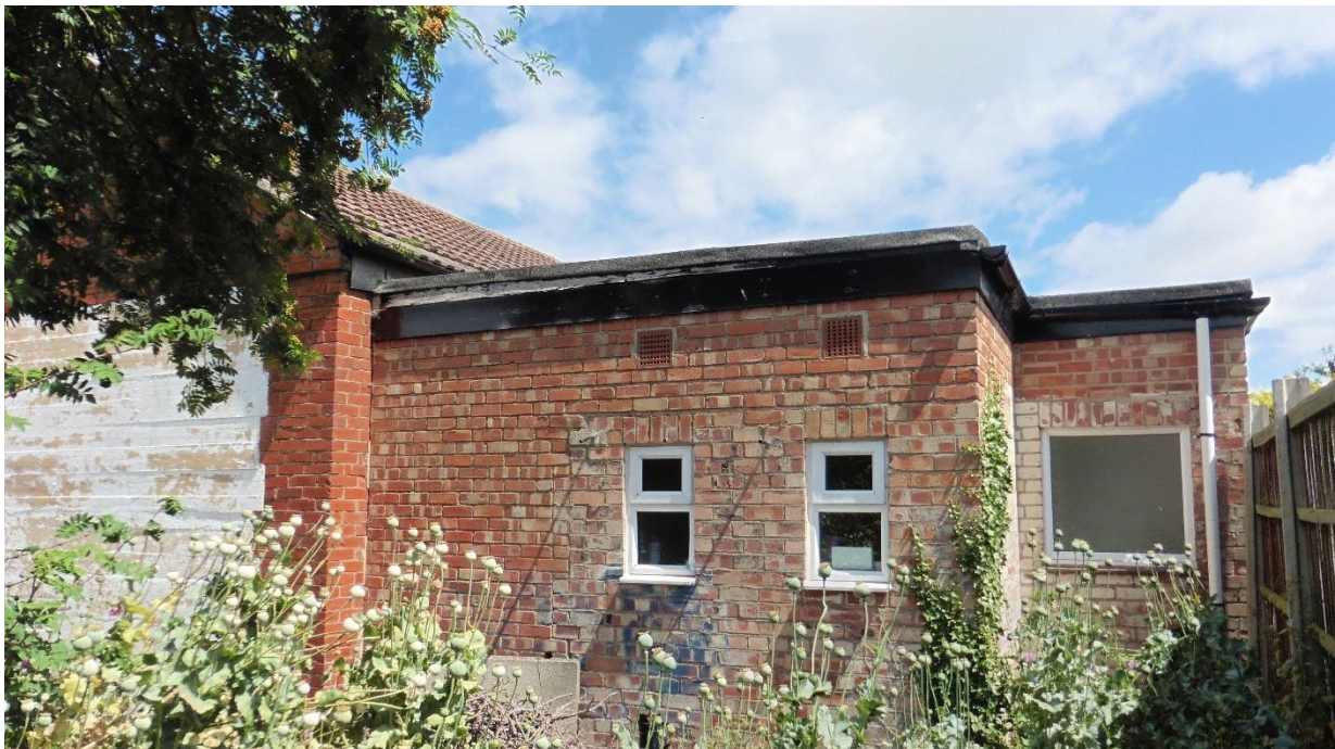
Photograph 2: Langar-cum-Barnstone Village Hall, taken from the south-west, showing the flat roof extension to the rear of the building constructed from cavity brick.
