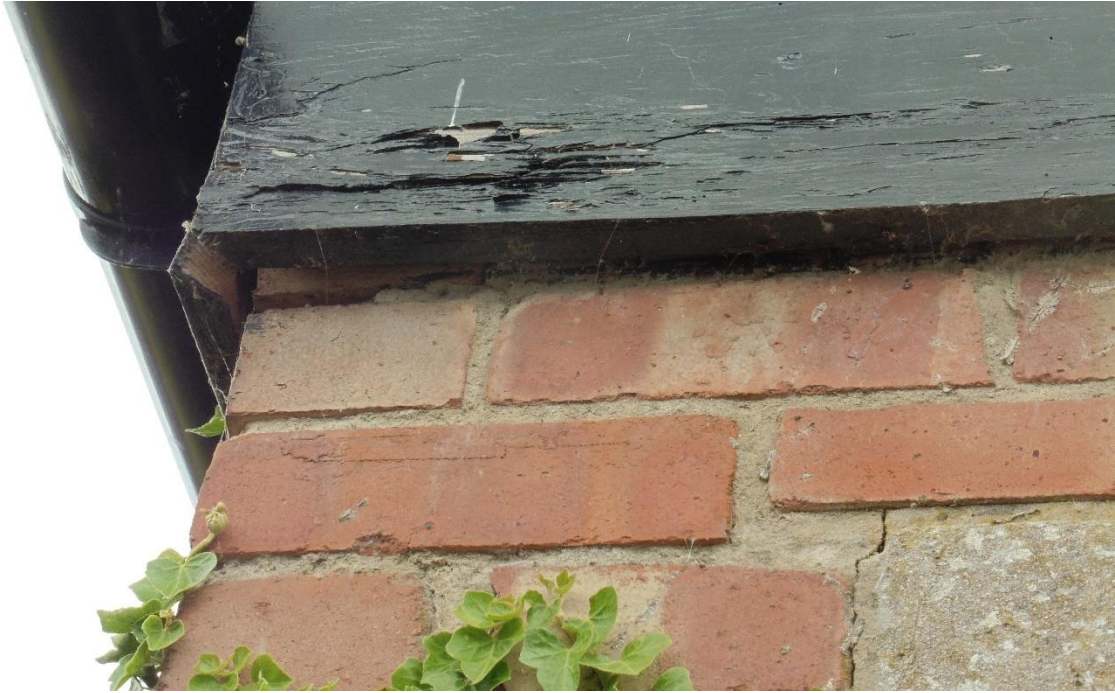
Photograph 7: Evidence of gaps behind the timber bargeboard on the south-eastern corner of the flat roof section.
