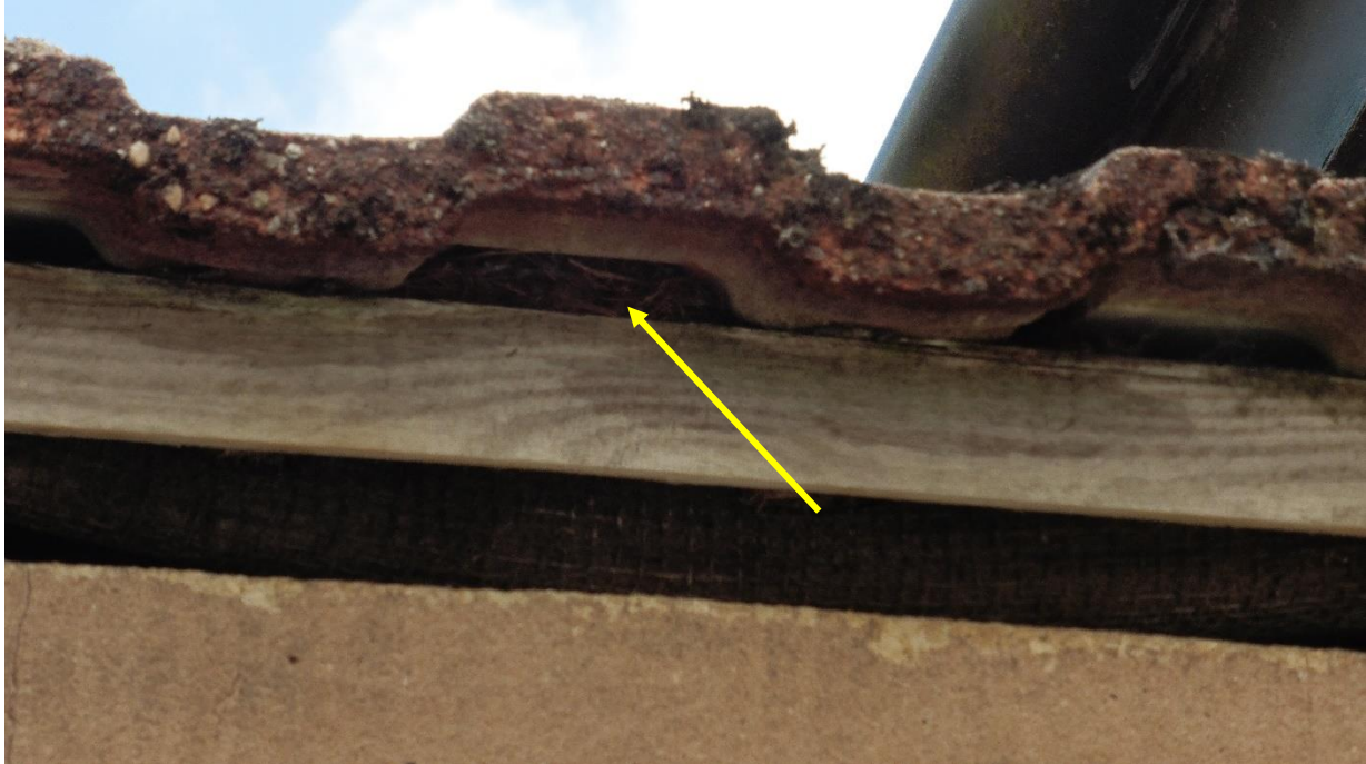
Photograph 9: Evidence of historic nesting material identified behind the bitumen felt within the void between stone and roofing material on the north facing porch.
