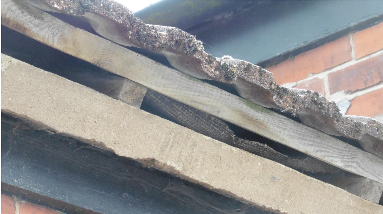
Photograph 5: Evidence of the void between the coping stone of the north facing porch and the roofing frame and bitumen felt underlining.
