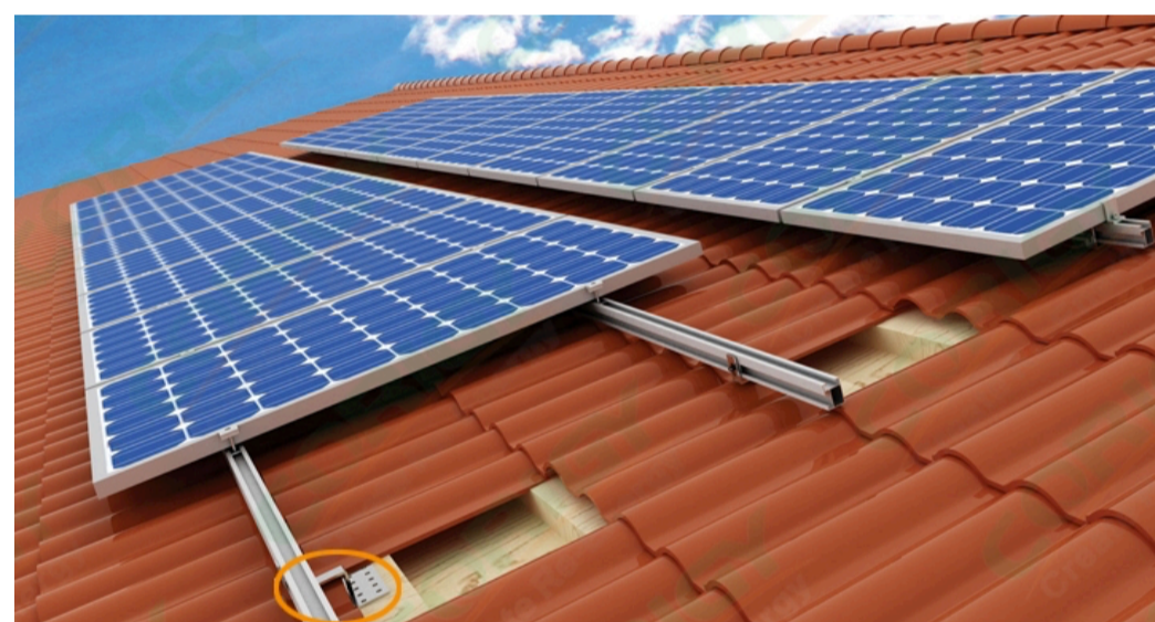
PHOTOGRAPH of PV panel installation
