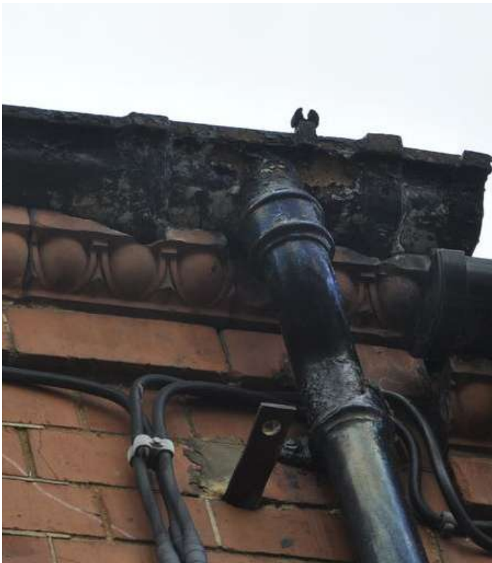
Damaged and leaking cast iron rainwater pipe
