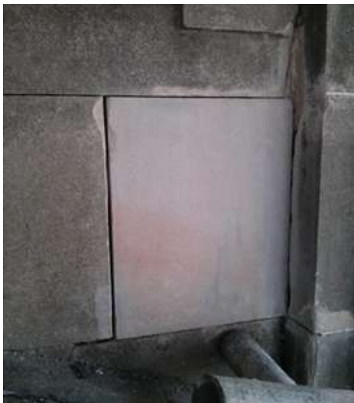
An indented stone having just been inserted in place. Pointing still to be done.
