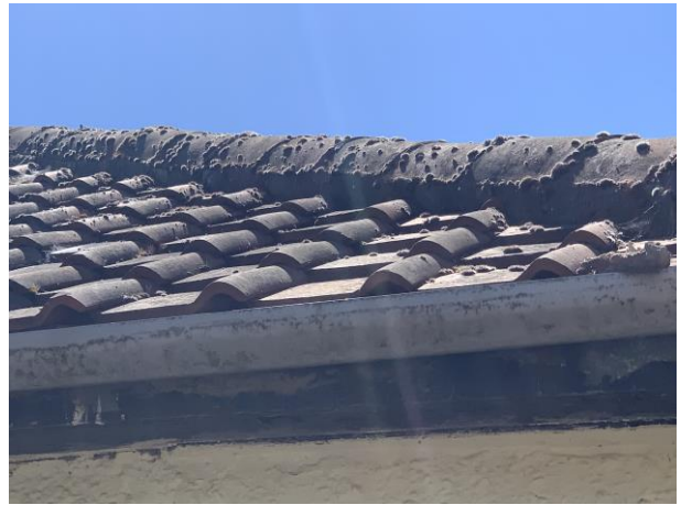
Photo 8: Building 1, tiles w/ house sparrow nest under (N)
