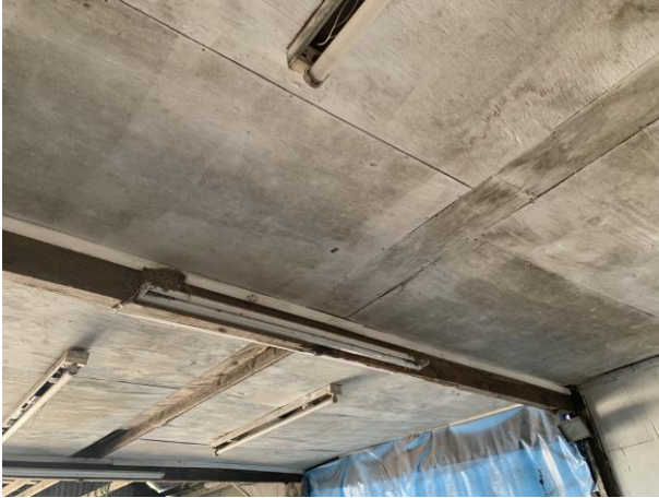
Photo 13: Building 2, old house martin/swallow nests.
