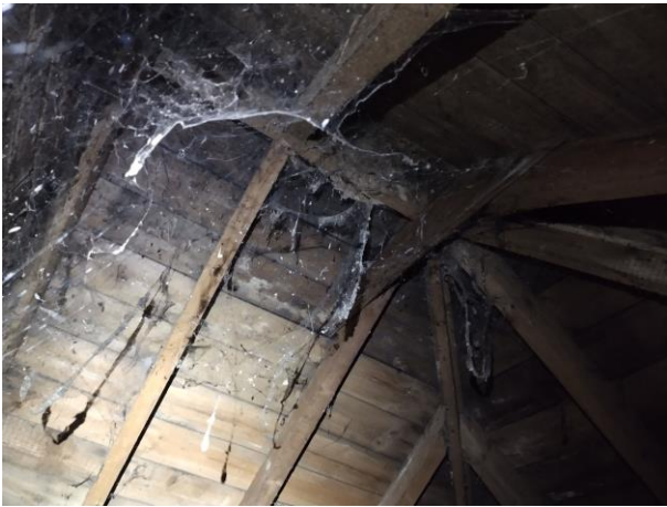
Photo 9: Building 1, loft void. Heavily cobwebbed.
