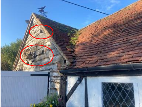
Photograph 1: Eastern gable with large gaps in timber weatherboarding and gaps in roof tiles (re-entry points circled)
