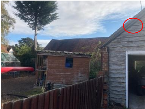
Photograph 5: View of western aspect, re-entry point circled
