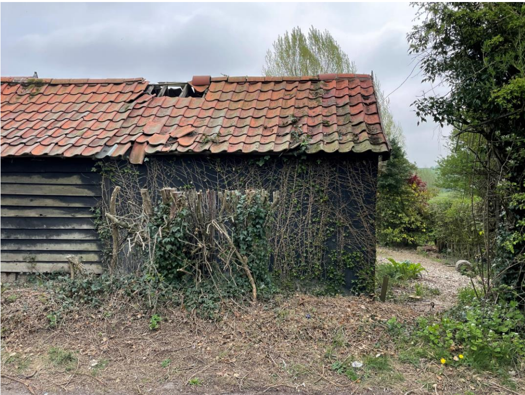
Area of roof damage and missing roof tiles to main barn
