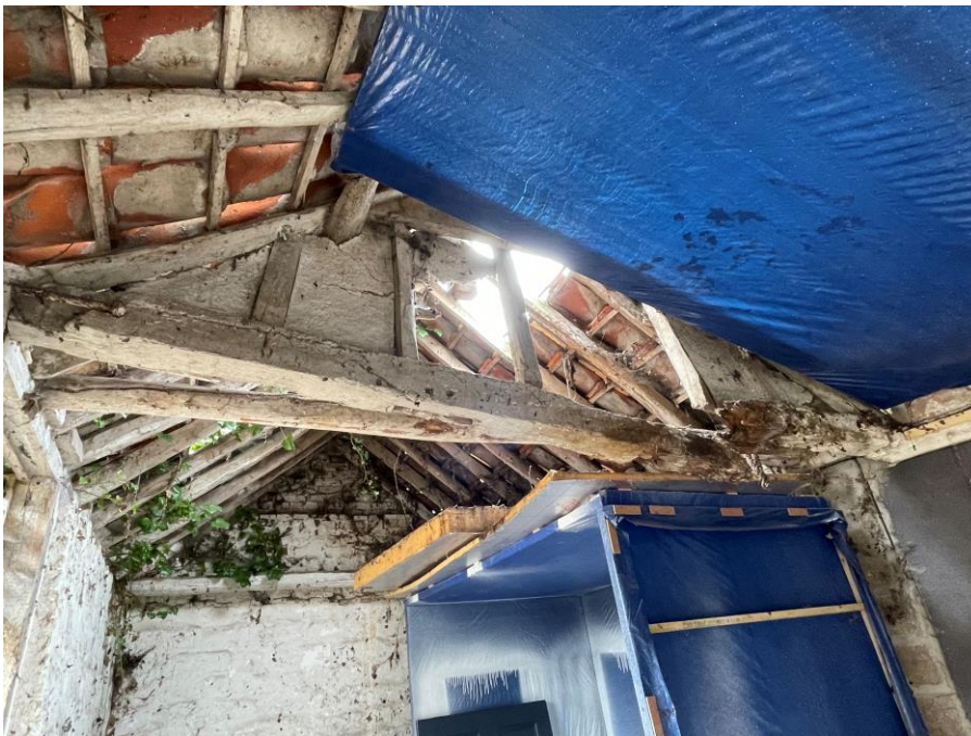
Figure 2 – Collapse to roof structure and missing tiles
