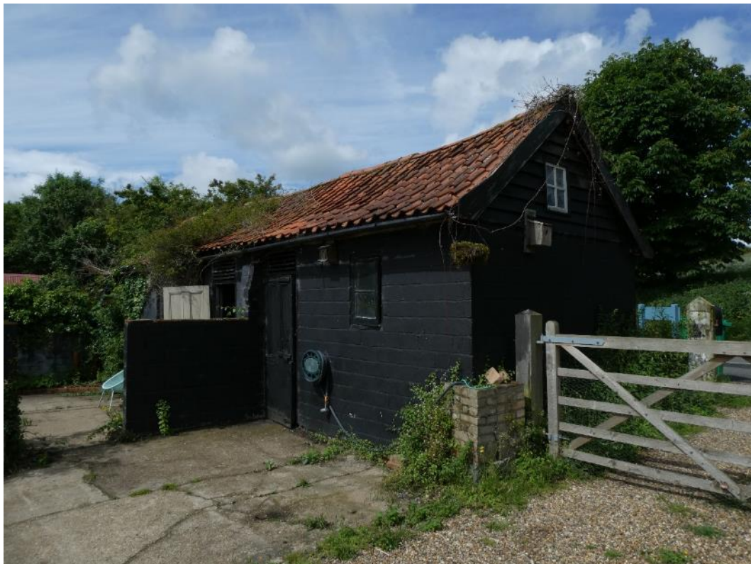
Photo 6 , building one external view showing breeze blocks, pantile roof and ivy cover, looking west.
