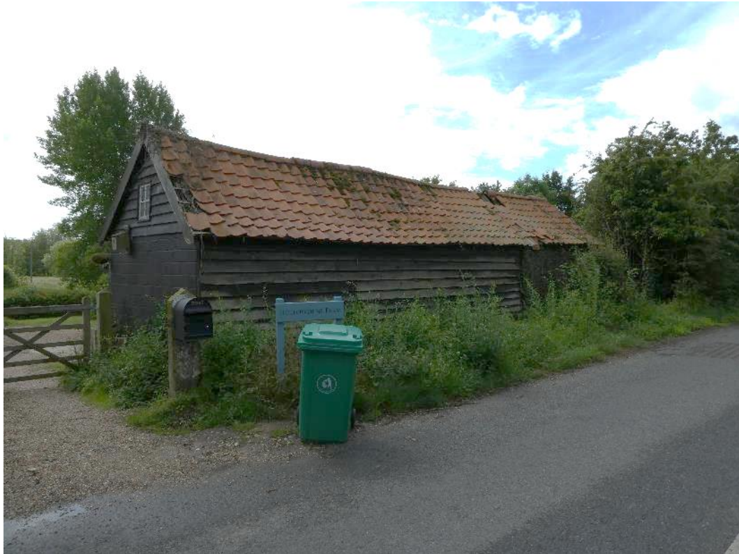
Photo 7 , external view of the weatherboarding along the north/northwest aspect of building one.
