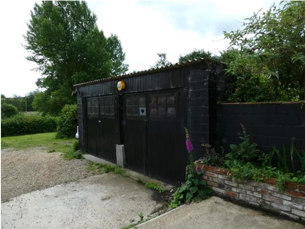
Photo 14 , external view of the garage (building two), showing broken glass window, facing southwest.
