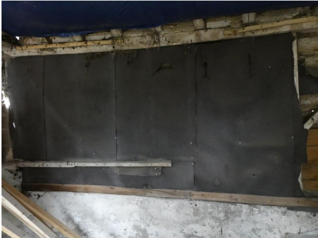
Photo 11 , bitumen covering an area of weatherboarding on the inside of the north aspect.
