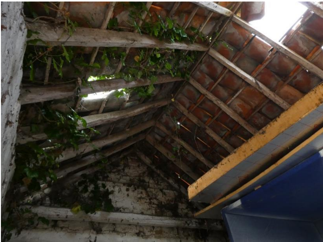
Photo 10 , internal view of the roof showing lifted and broken pan tiles with ivy ingress.
