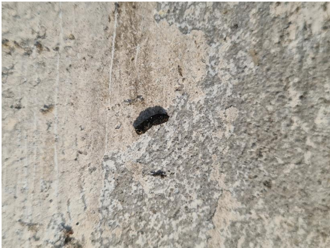
Photo 12 , bat dropping located on wall underneath bitumen.
