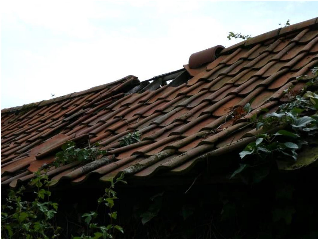
Photo 9 , external view of the roof showing lifted, broken and missing pantiles.
