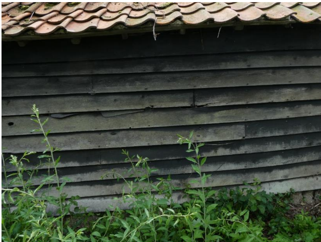
Photo 8 , example of weatherboarding on the north/northwest aspect of the building leading to a cavity between the bitumen felt creating a potential roosting opportunity.
