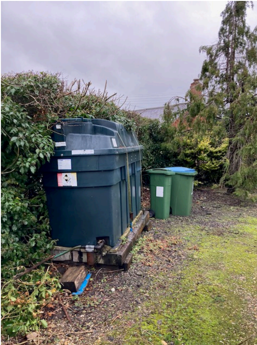
Fig 3: Existing old tank to be replaced with ASHP renewable energy system.
