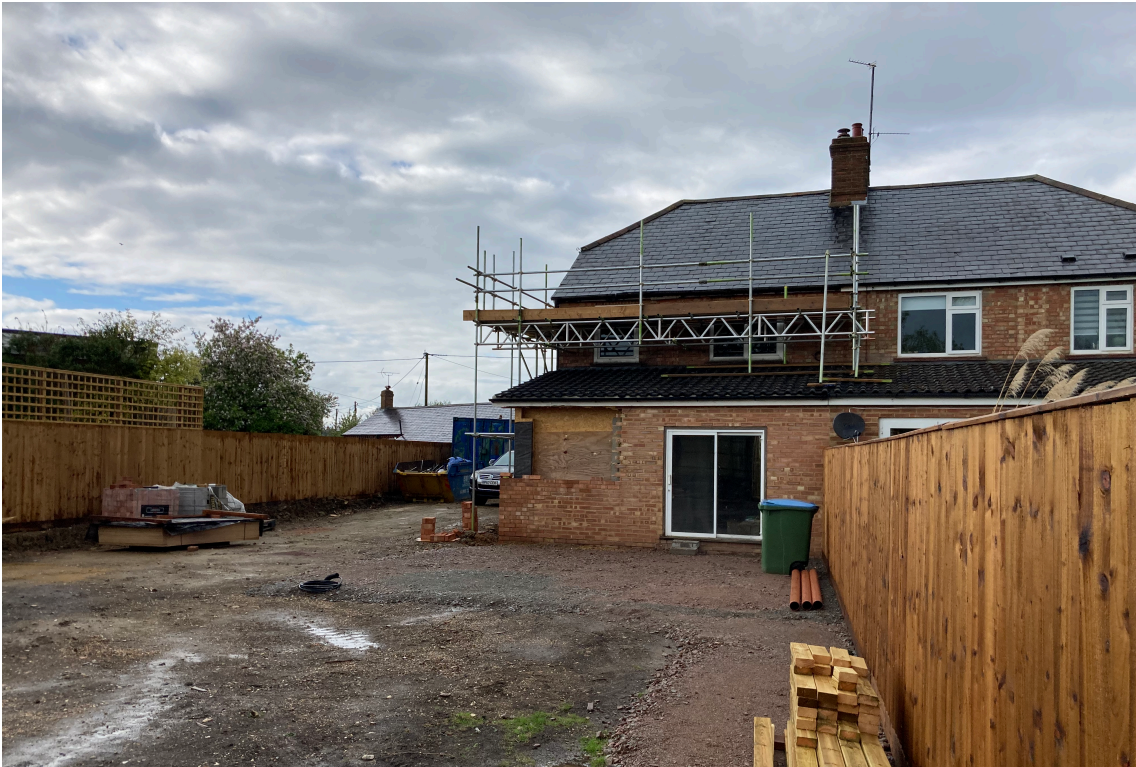
View of the rear following renovations of 8 Stock Lane - note the removal of the protruding rear extension, which is now inline with the gable of the house.
