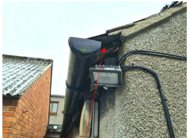
Figure 20: Outbuilding - gap at eaves under end tile.
