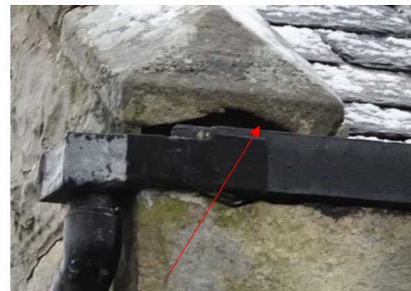
Figure 14: B1 - gap under water table of E gable end.
