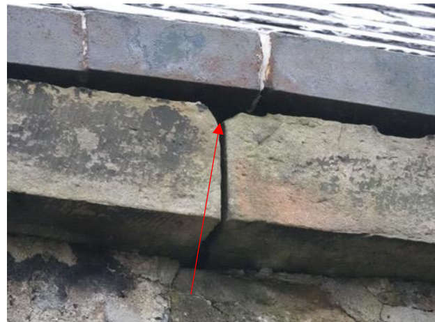
Figure 26: B1 - Gap in stone work at eaves of north elevation.
