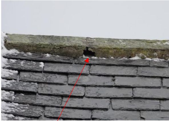
Figure 15: B1 - gap under ridge tile.
