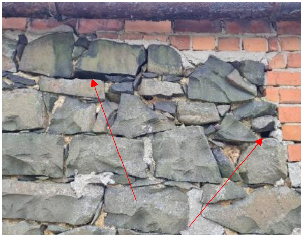
Figure 19: Outbuilding - gaps in the wall on NW elevation.
