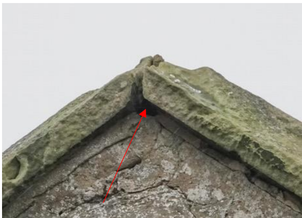
Figure 17: B1 - gap under end ridge tile on the N gable end.
