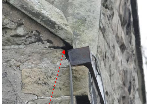
Figure 16: B1 - gap under water table on the W corner of north gable end.
