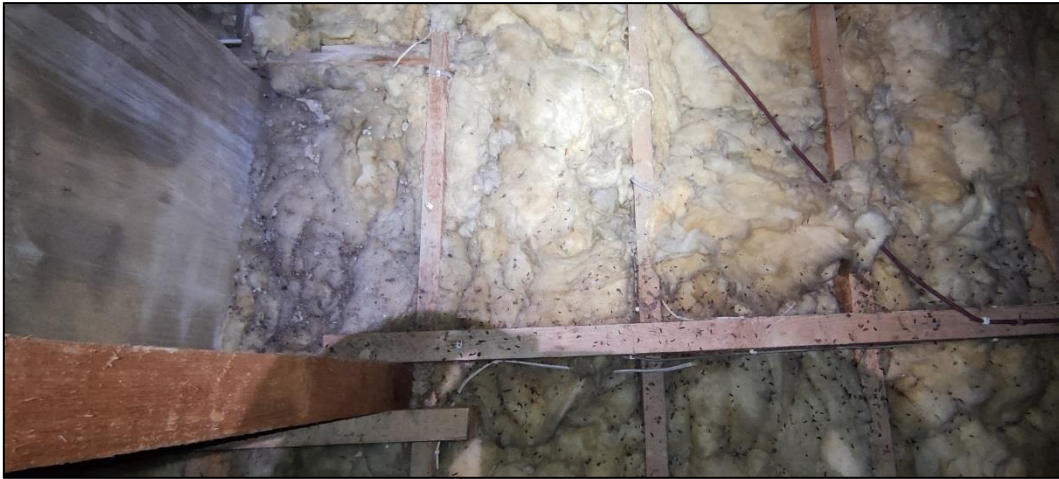
Figure 25 – more concentrated area of bat droppings close to a chimney stack
