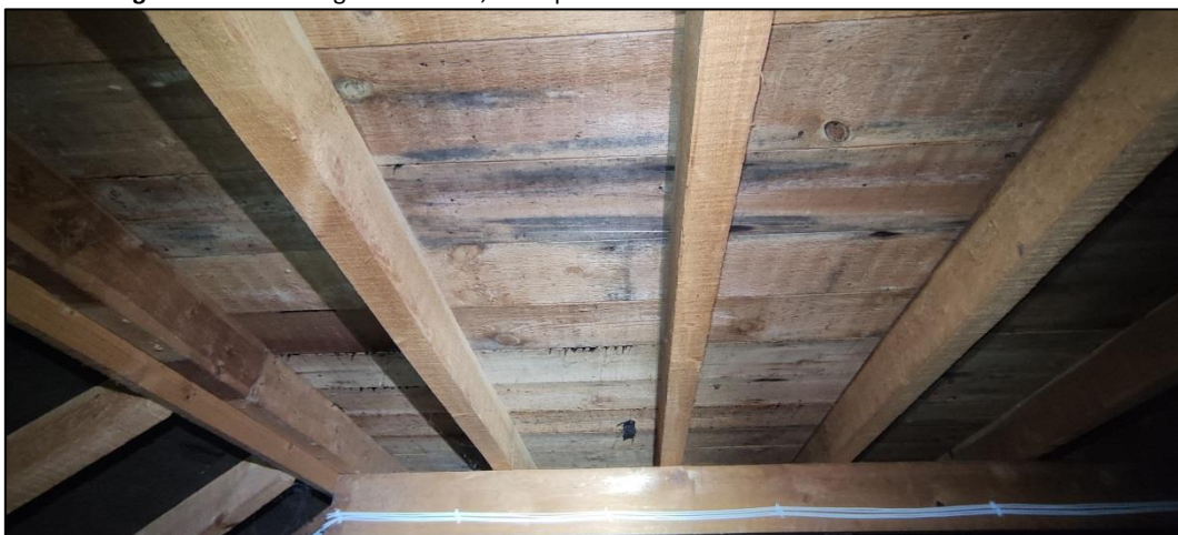
Figure 16 – showing underside of the flat roof section with sarking boards and pitch sealant
