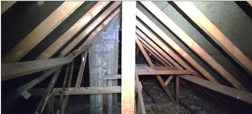
Figure 20 – showing one of the extended sections with rendered chimney in poor condition
