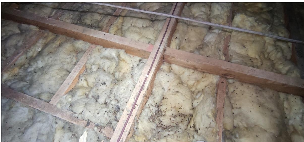
Figure 24 – scattered bat droppings throughout roof void 2
