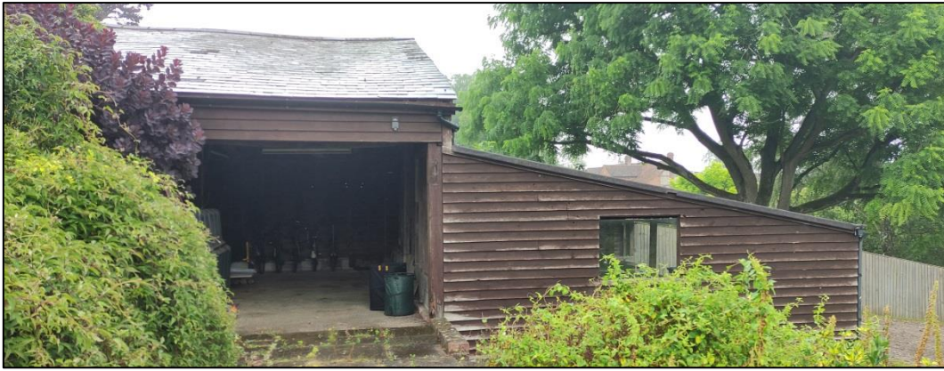
Figure 46 – showing open area where doors would have been and sloping bitumen roof
