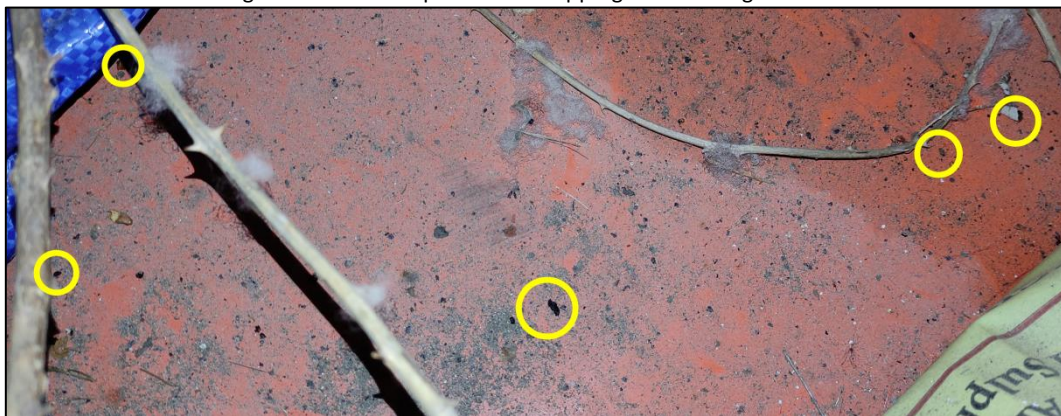
Figure 44 – bat droppings found at the southern end of the barn
