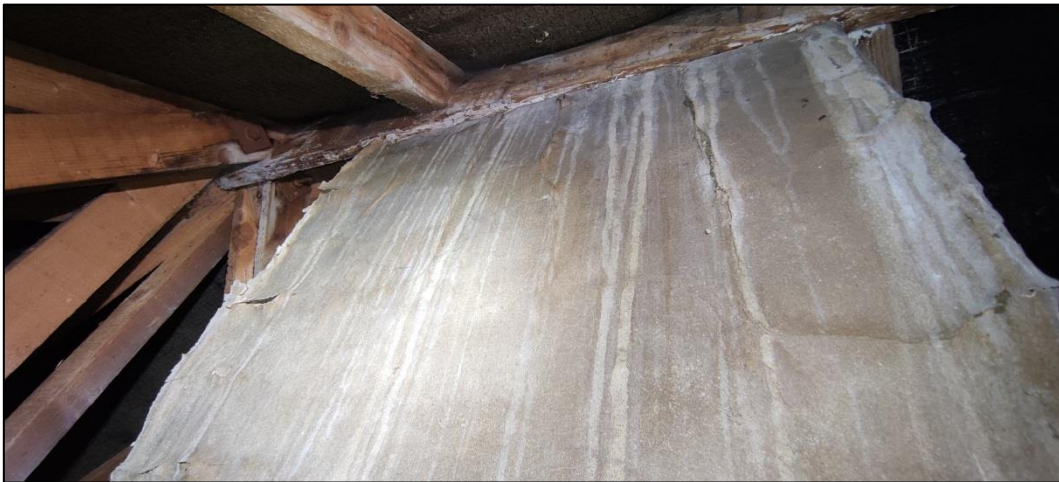
Figure 21 – Close up of flaking render on chimney stack and signs of water damage
