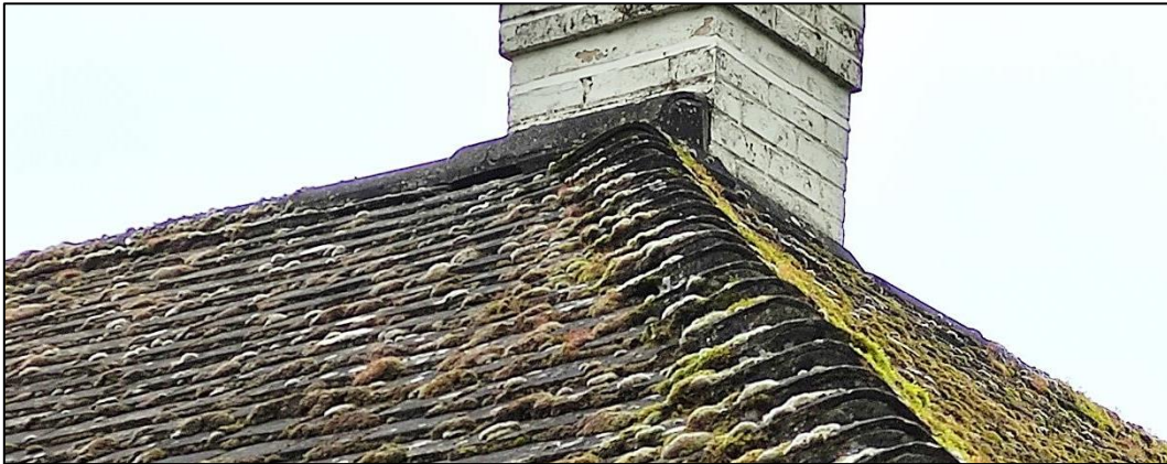
Figure 29 – image showing missing mortar and gap between ridge and chimney
