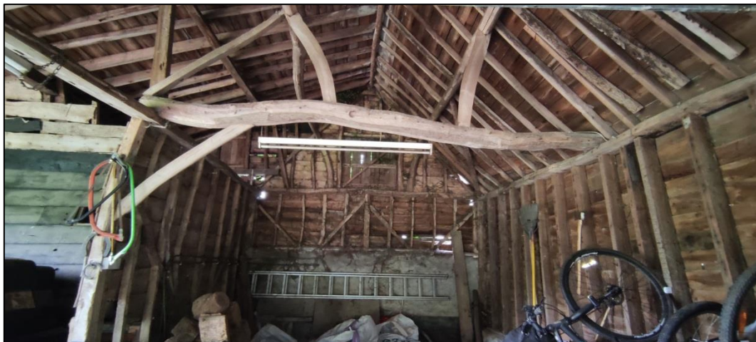
Figure 38 – showing hand-hewn timbers and holes in weatherboarding
