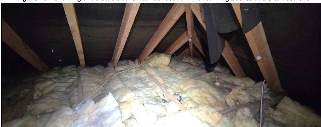
Figure 17 – showing sagging areas of bitumen felt underlay
