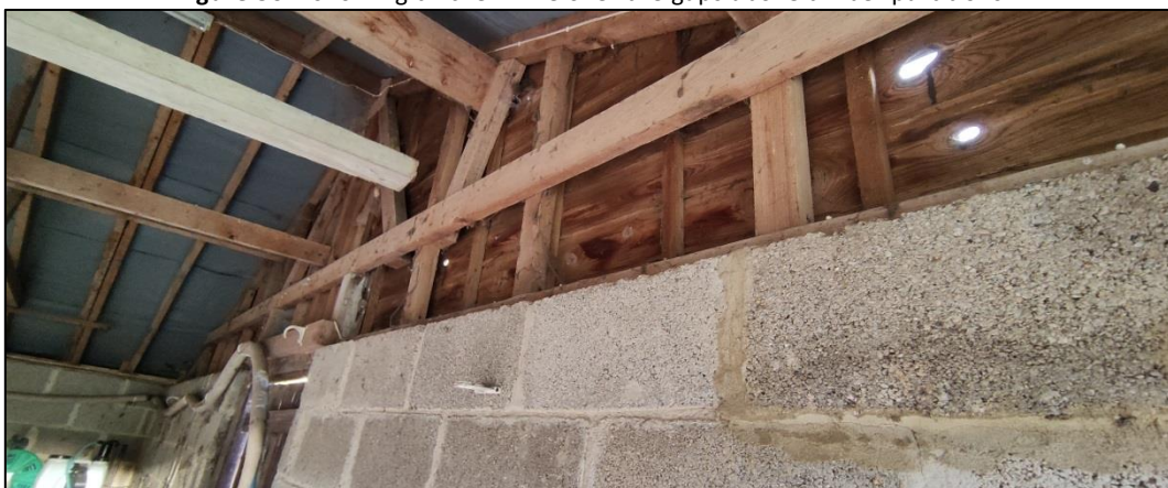
Figure 50 – showing breeze-block walls with timber weatherboarding with gaps throughout
