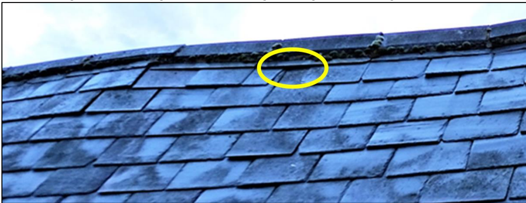
Figure 48 – gap where missing slate meets the ridge tiles
