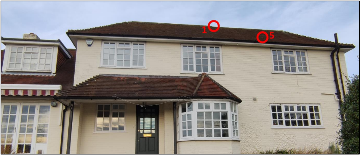
Figure 61 – Building 1 - Main House access points (circled) used by bats during the activity surveys at Orchard Cottage
