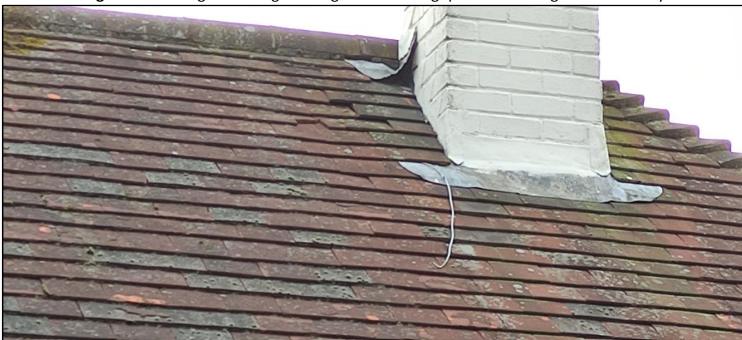
Figure 30 – image showing lifted tiles and lead flashing missing around chimney stack
