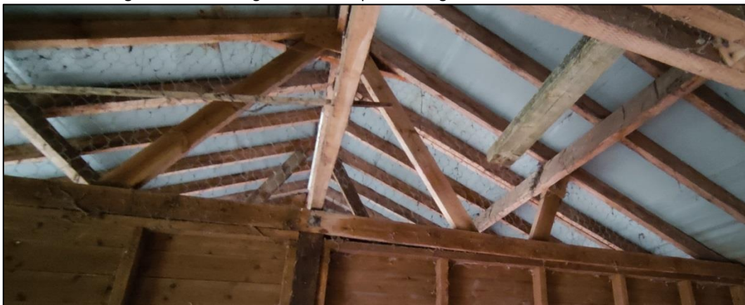
Figure 50 – showing chicken wire over the gaps above timber partitions
