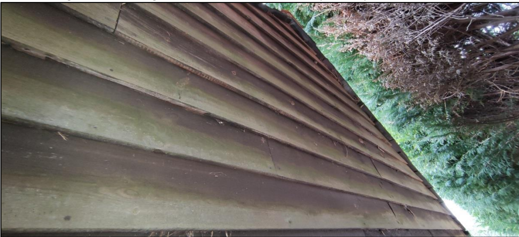
Figure 36– showing tightly fitting weatherboarding and proximity to trees
