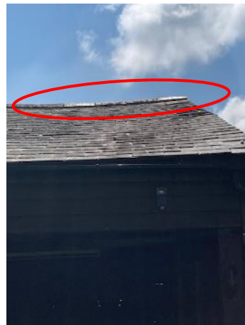
Figure 47. B5, gaps in mortaring of ridge tiles.
