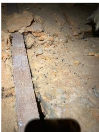
Figure 34. Scattered bat droppings, loft void 2, B1.
