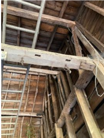
Figure 49. Interior of B5 showing wooden beam with shallow gaps on underside.
