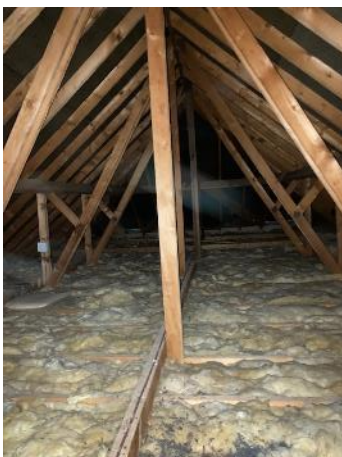
Figure 28. B1, loft void 1. Note bat droppings at bottom of picture.
