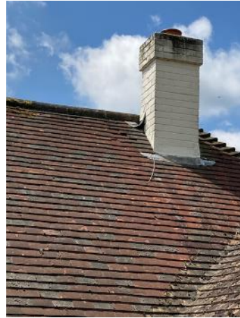
Figure 25. B1, lifted lead flashing around central chimney.
