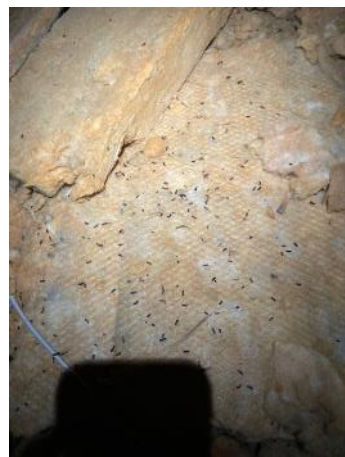
Figure 29. B1, loose aggregation of bat droppings under ridge beam.
