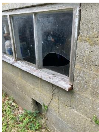
Figure 41. Broken window on south eastern aspect.
