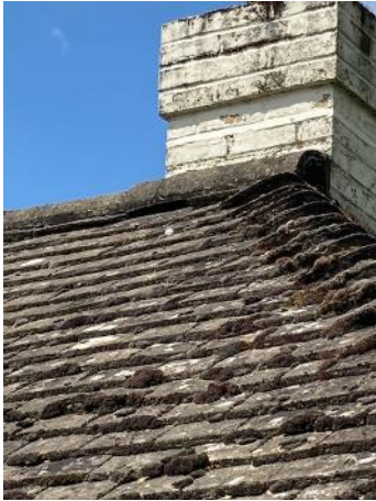
Figure 24. B1, gaps around ridge tiles.
