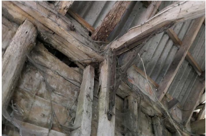
Figure 46 (right). Side bladed scarf joint and iron bracing to strengthen where a timber brace is missing.
