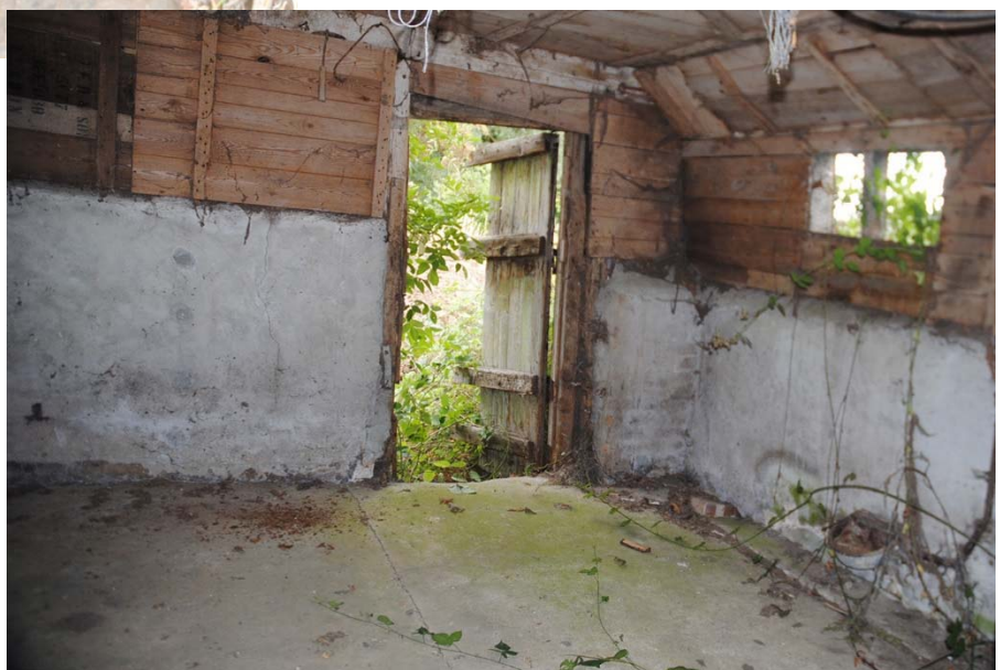
Figure 48 (below). The long C19 stable range, converted for use as calf pens by 1898. The structure where not covered by concrete block and boarding, appears lightweight. (see left).
