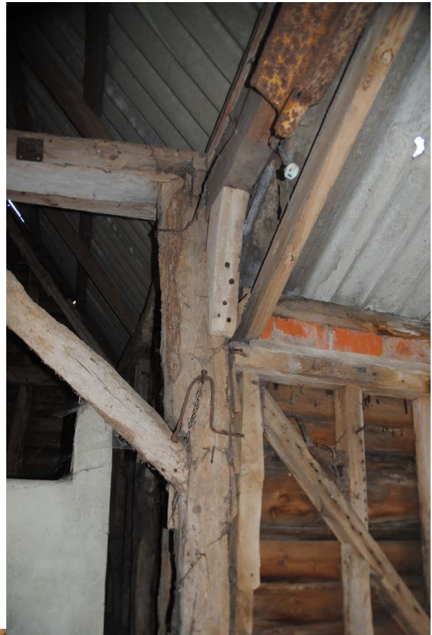
Figure 43. Typical jowled post, at the junction with the midstrey. This shows reused timbers and predominately nailed joints, indicating a C19 date for the braces. The midstrey (right) is butted later onto the side of the main structure.
