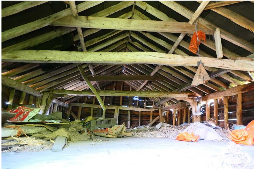
Figure 52 (right). Barn 2 interior. Upper floor showing late C18/early C19 structure and roof.
