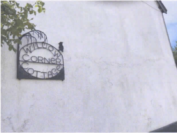
Photo 28: E elevation, cracked render
