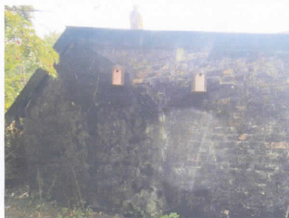
Photo 19: garage, N side, clay lump in E part (below gable) and brick in W part
