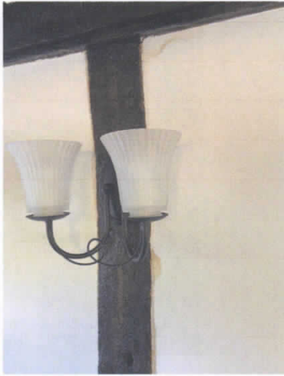
Photo 26: study, damp on E wall
