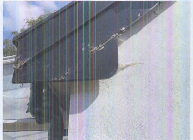
Photo 35: NW corner of garden room, rotten timber
