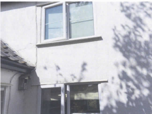
Photo 30: S elevation, cracked render
