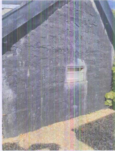
Photo 21: garage, glazing missing on S side
