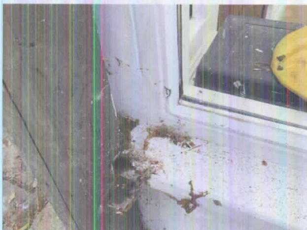
Photo 36: N side of conservatory, rotten timber
