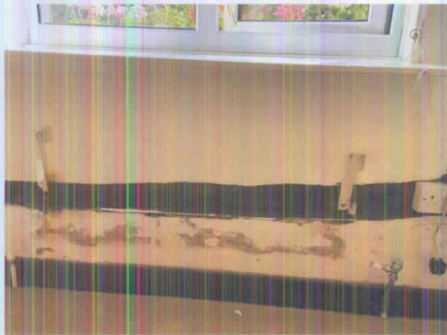
Photo 22: study, damp below sole plate on S side
