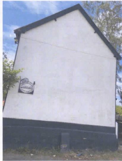
Photo 27: E elevation, cracked render
