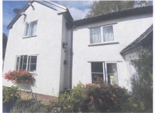
Photo 29: S elevation cracked render (gable is 20C, E of gable is 16C, 20C porch just seen on R)
