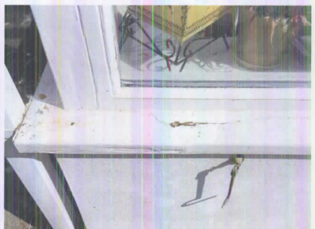
Photo 37: W side of conservatory, rotten timber
