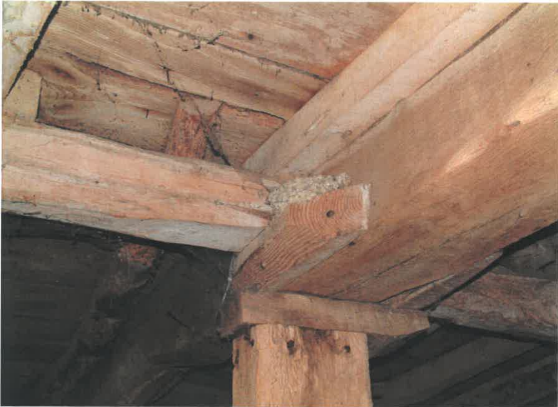
One of the oak Samson posts supporting the inserted floor made of various second-hand timbers
