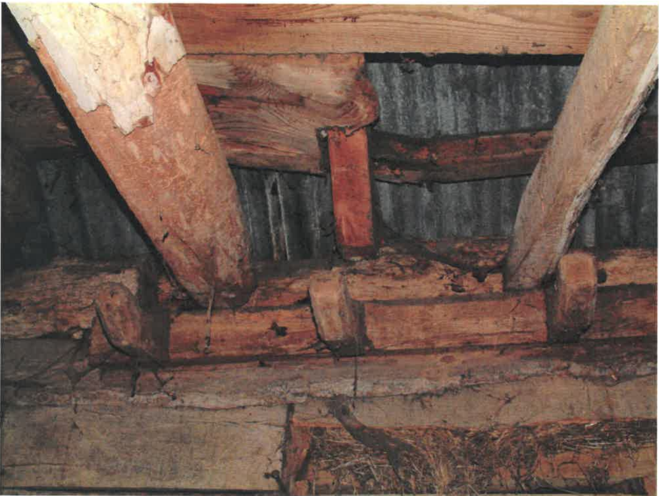
Some of the original timber hooks along the front wall, which have been compromised by the inserted floor
