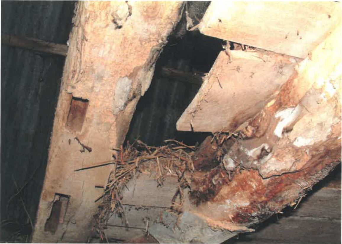
Decayed re-used timbers at the northern end of the inserted floor
