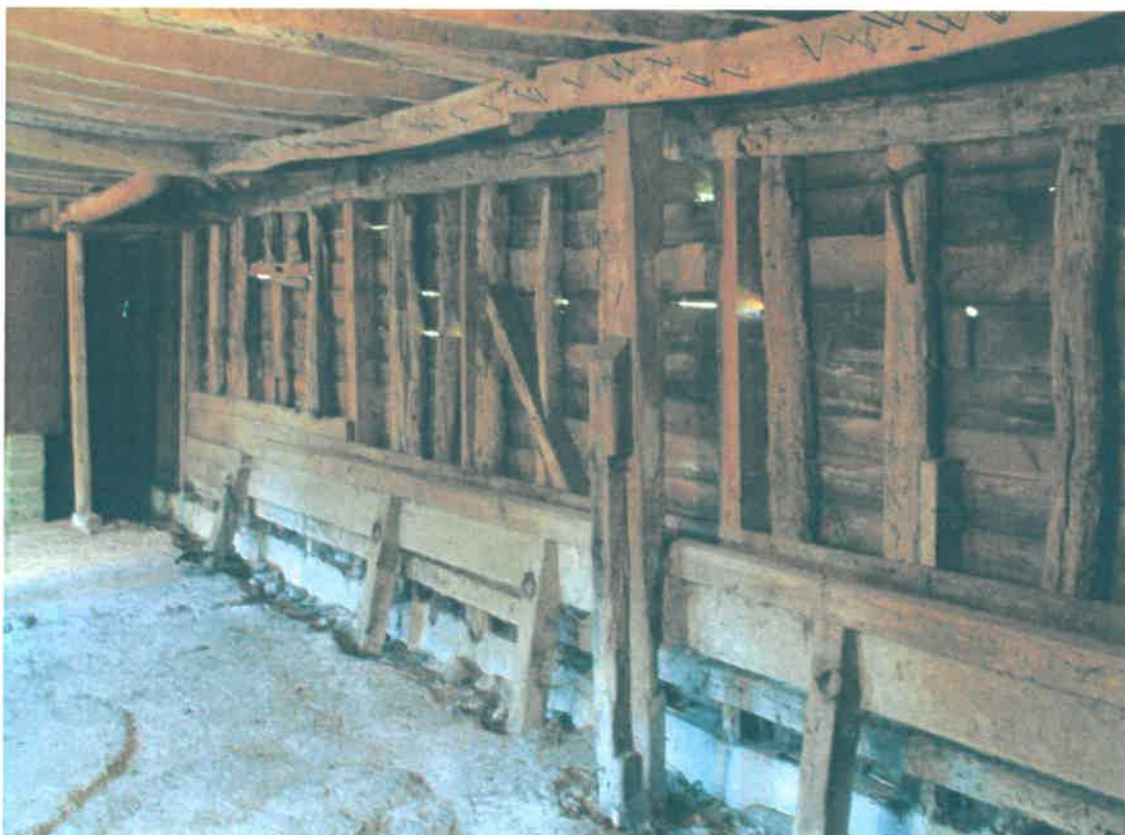
Part of the rear wall showing the original framing and inserted floor
