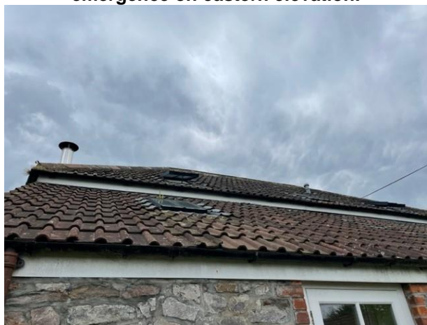
Photograph 4: Gaps under lead flashing.
