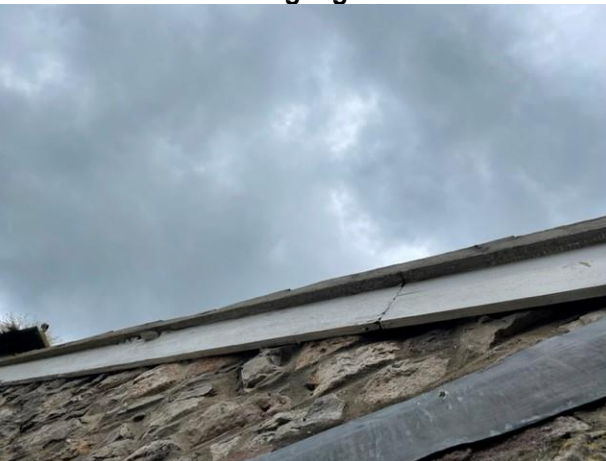
Photograph 5: Example of roosting feature under fascia boarding.
