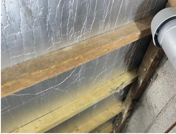
Photograph 7: Inside roof void on western end of the property with view of insulation.
