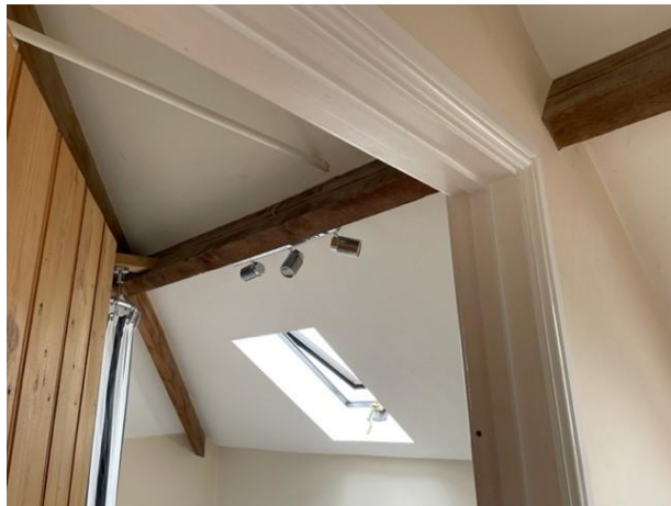
Photograph 6: Interior of house showing no roof void on extension.
