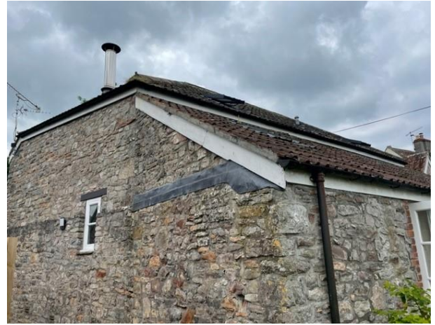
Photograph 2: East elevation with gaps in fascia boarding.
