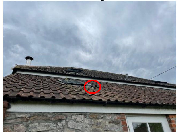
Photograph 4: Gaps under lead flashing.
