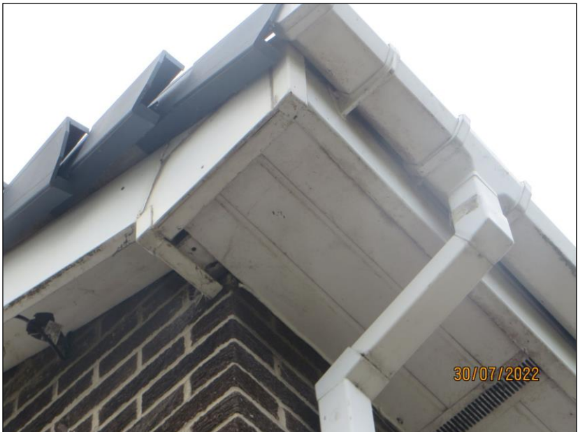
Figure 12. Gaps into soffit boxes and plastic cap tiles.
