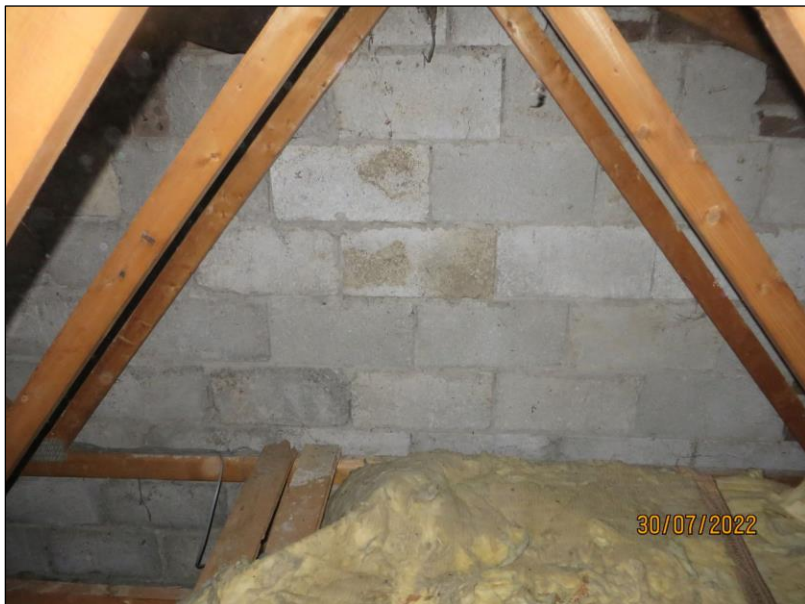
Figure 15. Wall with droppings present in the loft void.
