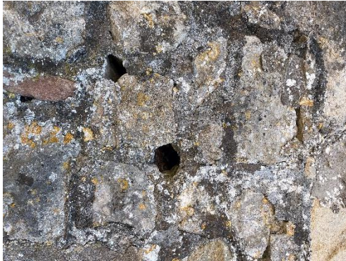
Plate 3: Gaps in Walls
