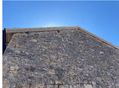
Plate 4: Gaps Behind Fascia Boards
