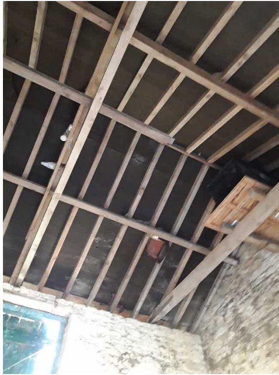
Photograph 3 – Tears in the roof lining of the former agricultural building
