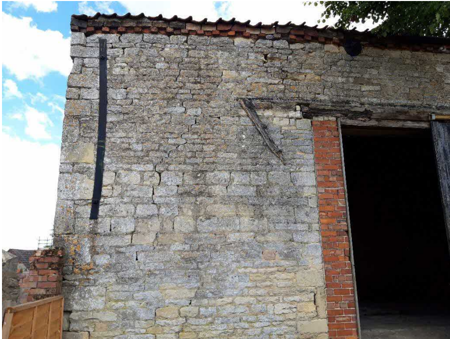
Photograph 4 – Absent mortar within brickwork of former agricultural building
