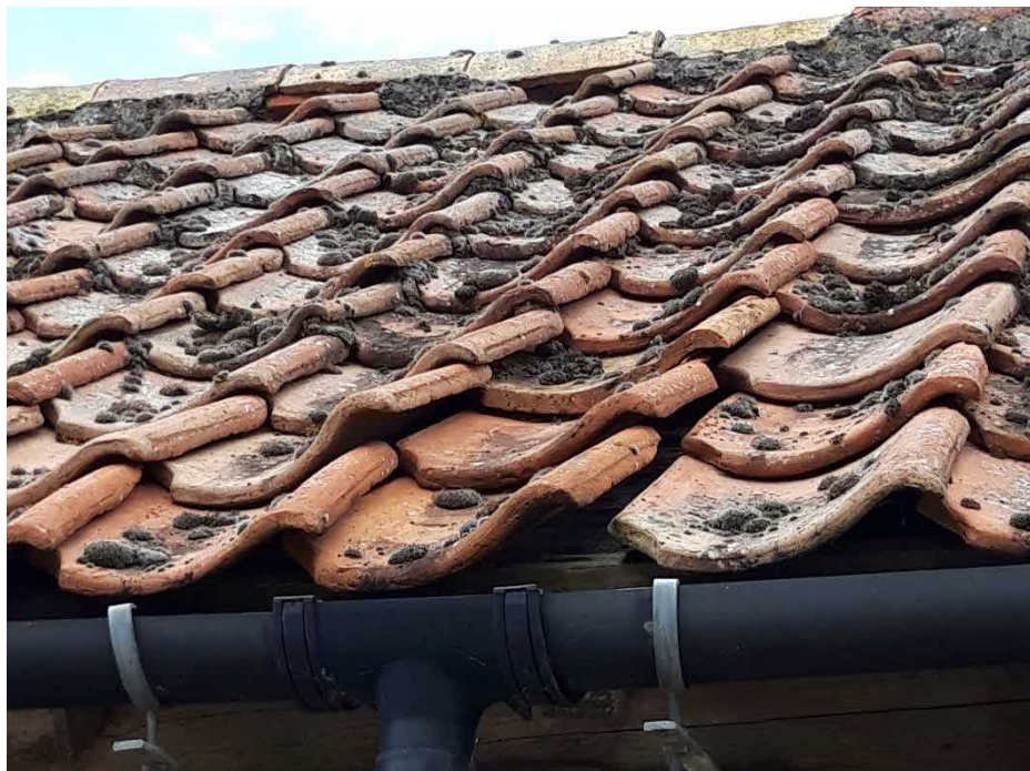
Photograph 2 – Lifted pantiles along exterior of former stable/cart shed
