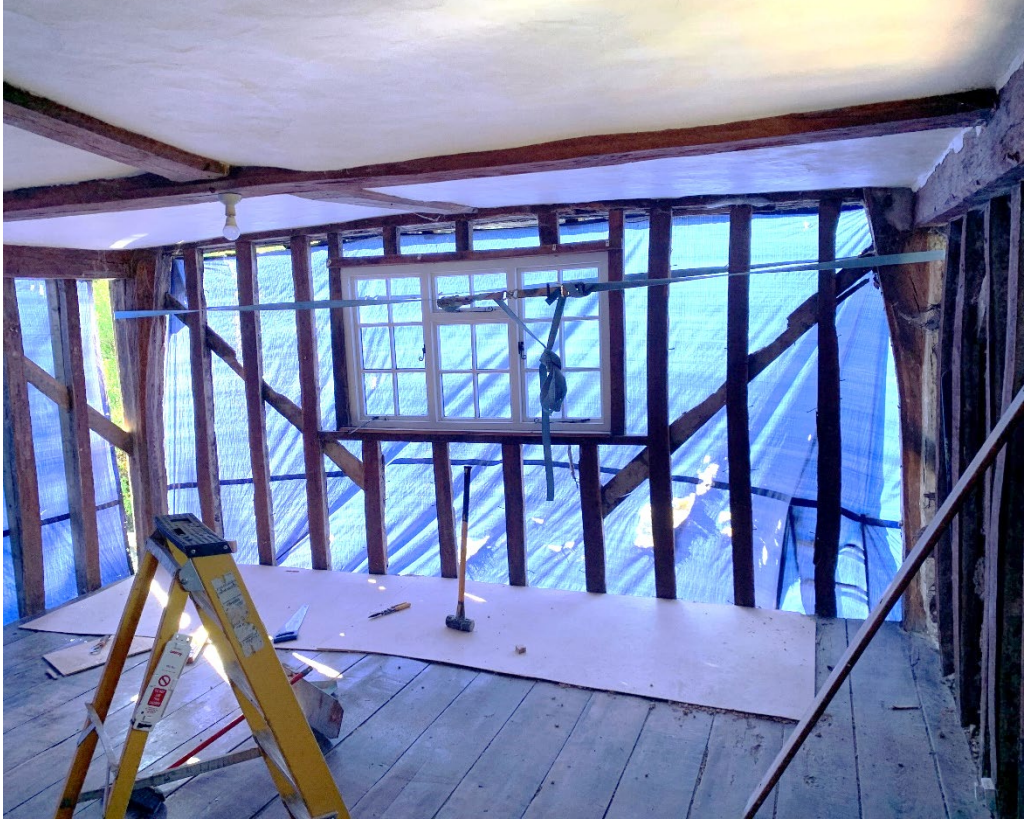
Figure 13: First floor parlour chamber showing the timber-framed structure of the parlour block.
