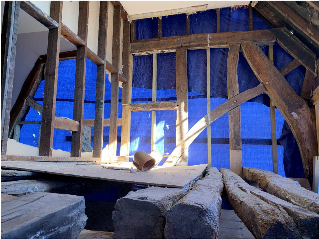
Figure 9: Serpentine windbracing and an original window with rebate for shutterslide evident in the north end wall.
