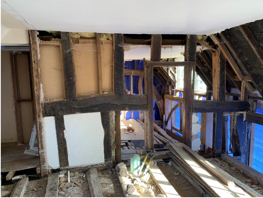
Figure 7: Upper closed truss between the service chamber/loft and the former open Hall. Jowled post to right.
