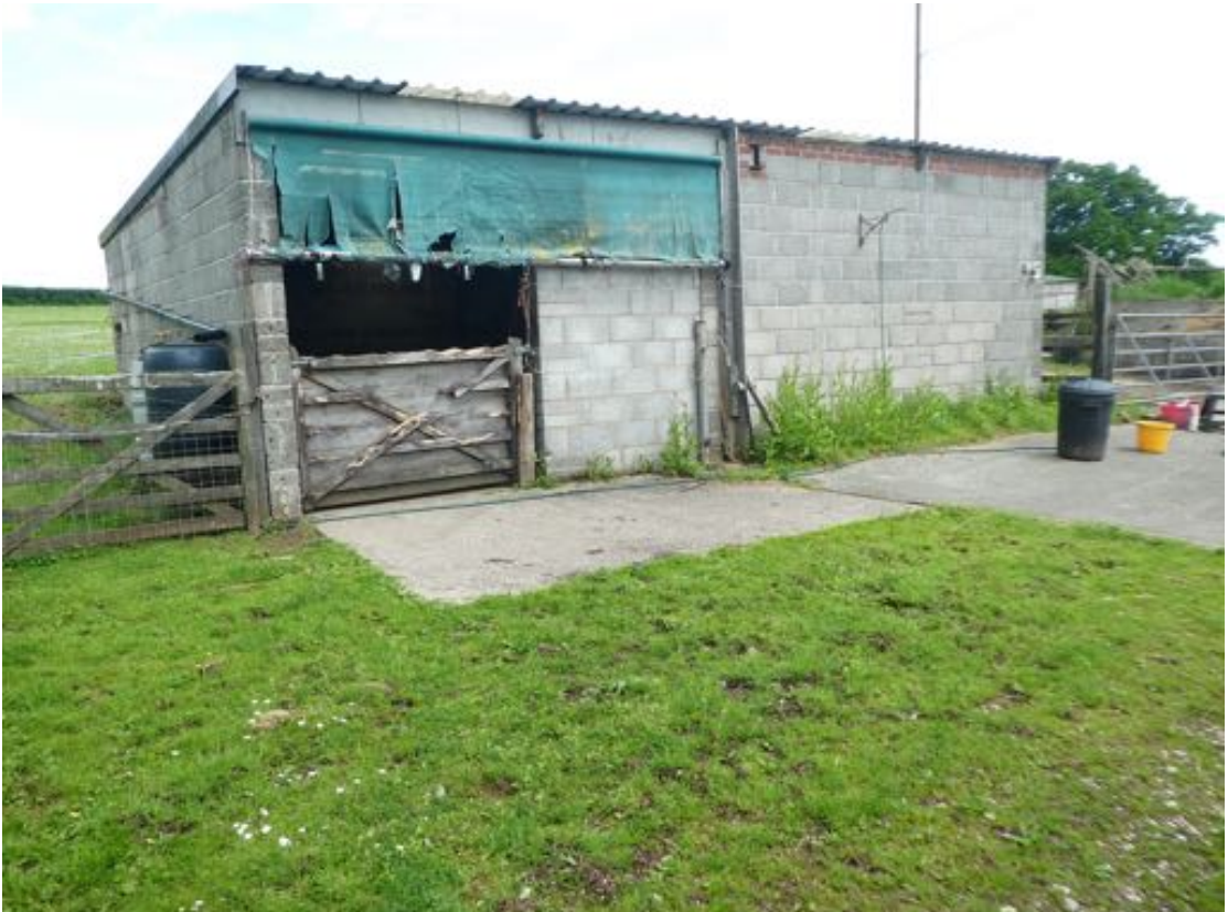
The western side of the stable/barn is shown in this image, with the barn part behind the gate and the green screen. A corrugated plastic panel set into the roof provides an abundance of natural light in the barn part. Both sides of the single floor area building are very well ventilated as well as well lit
