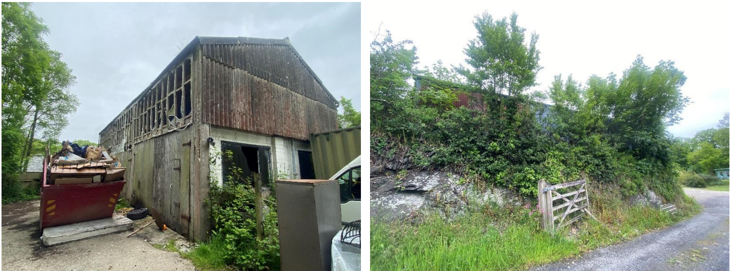
Figure 1: The southern aspect and western end (left) and the northern aspect of the building behind a hedgebank (right).
