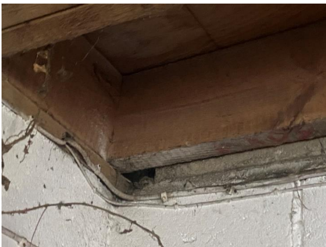
Figure 6: An example of the gaps at the wall top in the western room providing access to a cavity wall.
