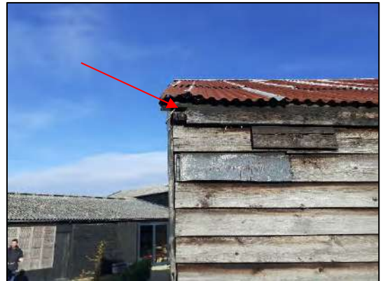
Photo 14. Gap in outer wall of Building 2
