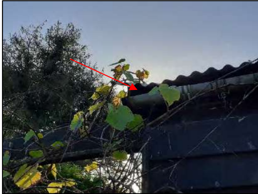
Photo 11. Gap between corrugated iron and outer wall of Building 2
