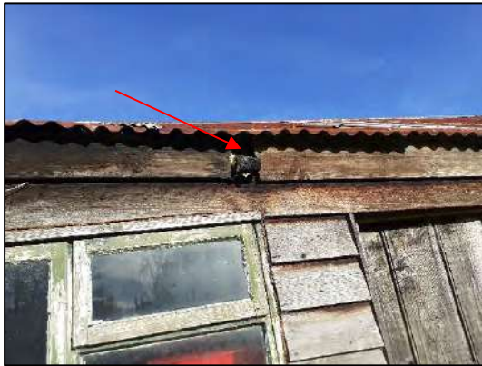
Photo 15. Gap in outer wall and insulation of Building 2
