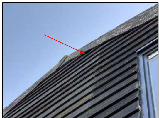
Photo 4. Gap in the roof of Building 1
