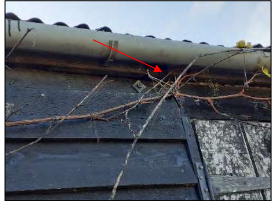
Photo 12. Gap in outer wall, roof and insulation of Building 2
