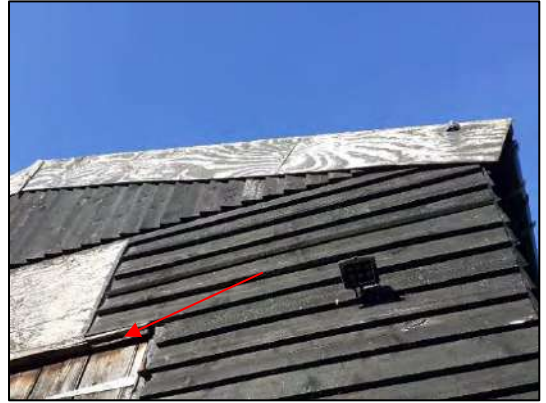
Photo 6. Gap in the door frame of Building 1
