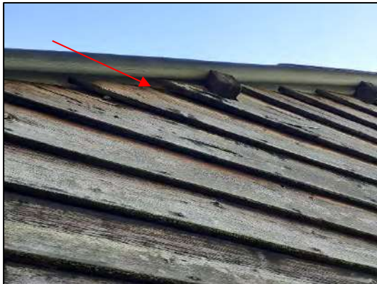
Photo 13. Gap between corrugated iron and outer wall of Building 2
