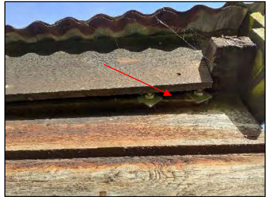
Photo 16. Gap in outer wall of Building 2
