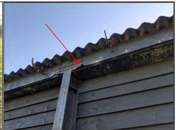
Photo 2. Gaps in the roof of Building 1
