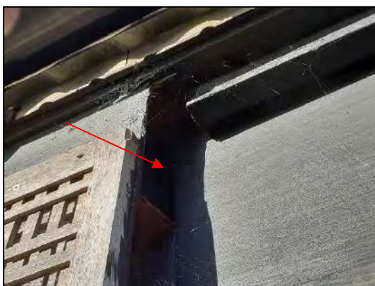
Photo 9. Gap in the roof panel of Building 1
