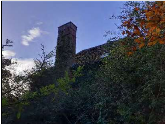
Photo 17. Building on neighbouring property with loose tiles and ivy
