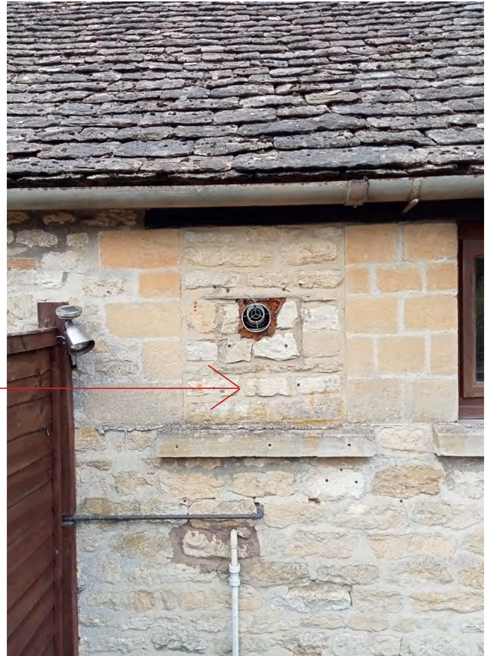
Cottage's window blocked up around boiler's flue
