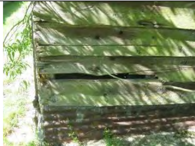
Gap in cladding on building 5
