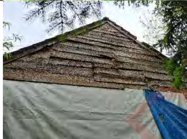
Large gaps in cladding on Main Barn.
