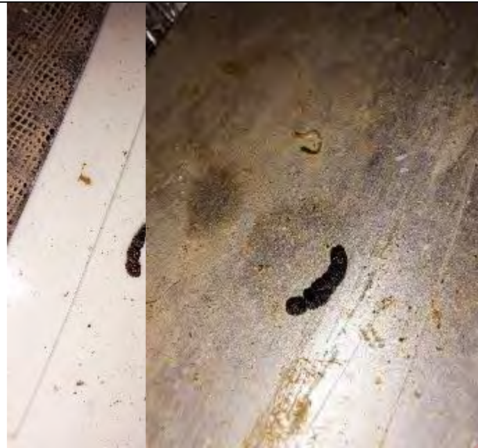
Bat droppings noted throughout.
