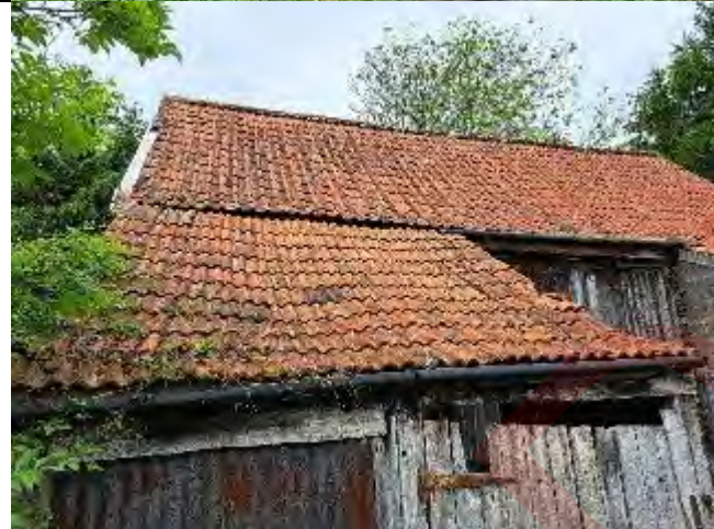
Gap above door to building 4
