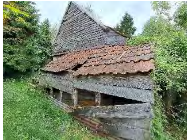
Large holes in cladding on building 3
