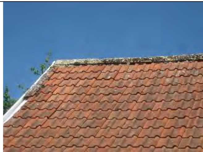
Gaps beneath the ridge tiles
