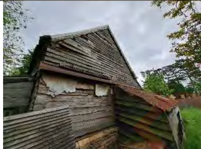
Holes in gable end on south-western side of the building
