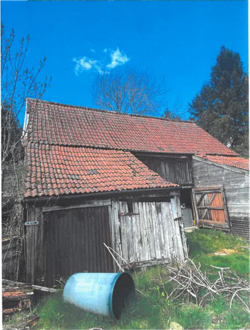
Front roof on left side again in very good alignment to main Barn
