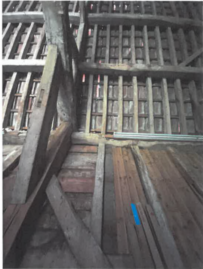
View on underside of roof within Barn, note substantial truss and purlins
