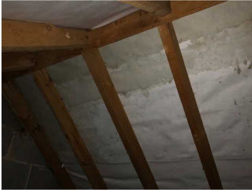
Plate 27. Extensive bat urine staining at northern gable end of Loft 1
