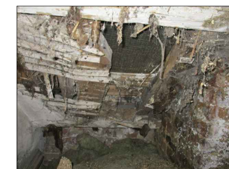
PHOTO TAKEN THROUGH ACCESS PANEL (WEST HIP)
