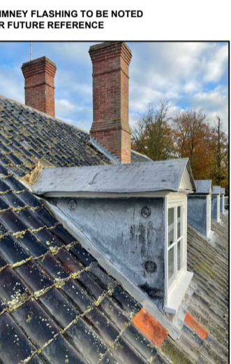
CHIMNEY FLASHING TO BE NOTED FOR FUTURE REFERENCE
